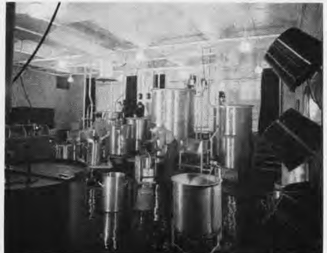
CONTROLLED CHEMICAL MIXTURES ARE PIPED TO PROCESSING ROOMS
