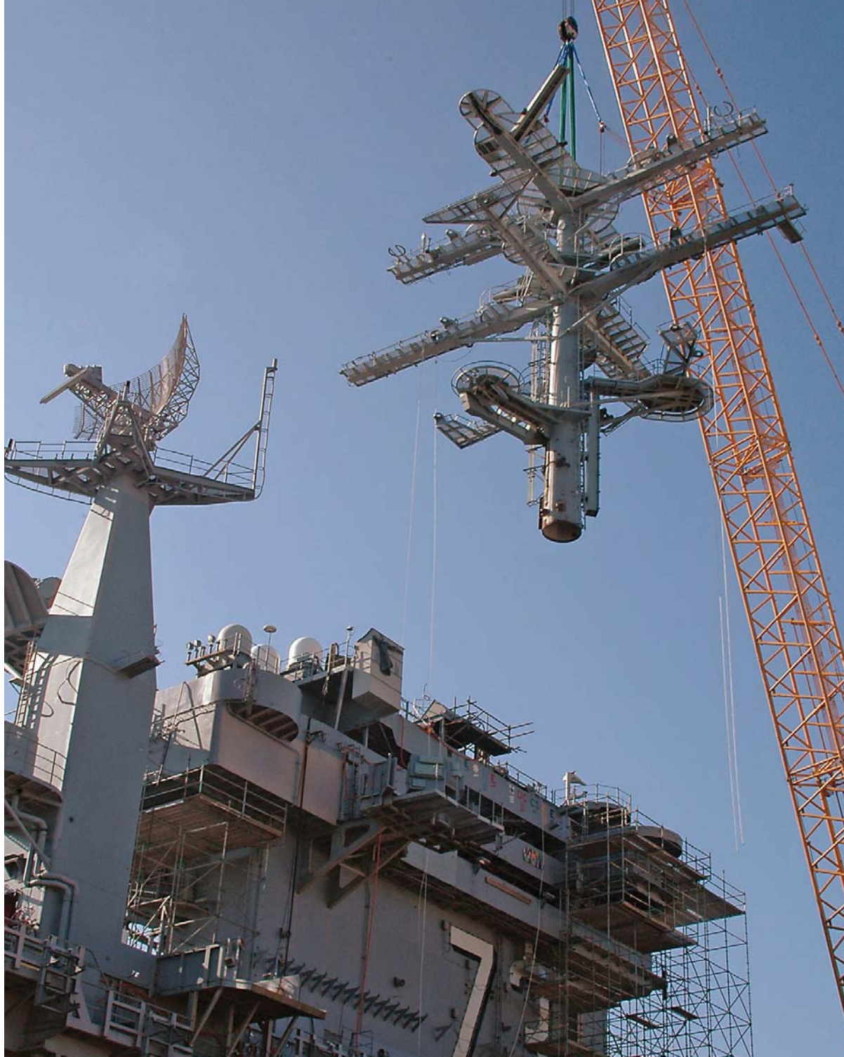
A crane removes the main mast from George Washington (CVN 73) during the carrier's shipyard availability at Norfolk Naval Shipyard in Portsmouth, Va., on 10 November 2006. Photo by MCSN Jennifer Aspey.
