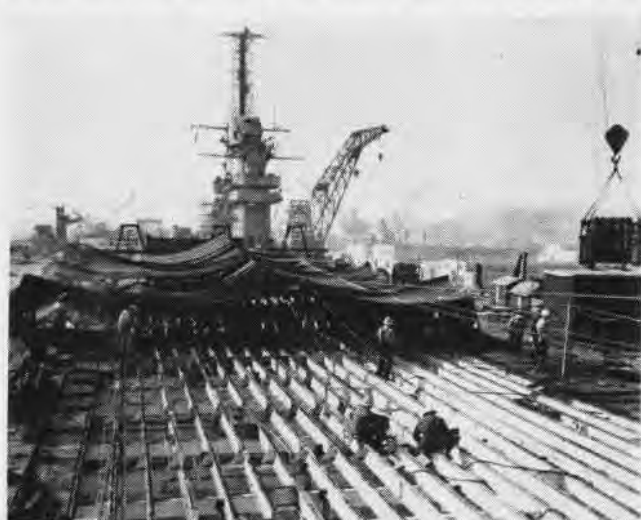
FLIGHT deck looks like an unfinished attic during preparations for laying steel deck on after end of the Kearsarge .
