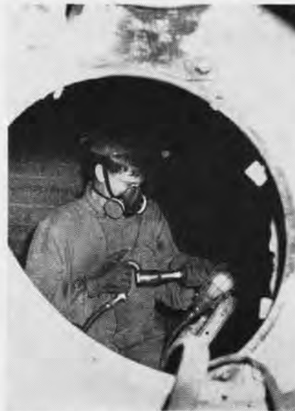
CHIPPING in subsurface boiler room makes confined quarters for SN Lloyd Burrows.
