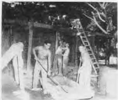
SEABEES prepare masonry for the new dependent housing project at Sangley Point.
