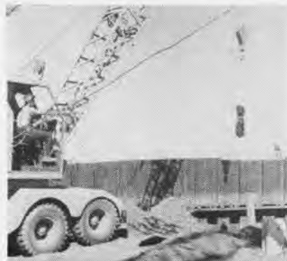
UNEXPLODED WW II bomb is gingerly hoisted while building new seaplane ramp.
