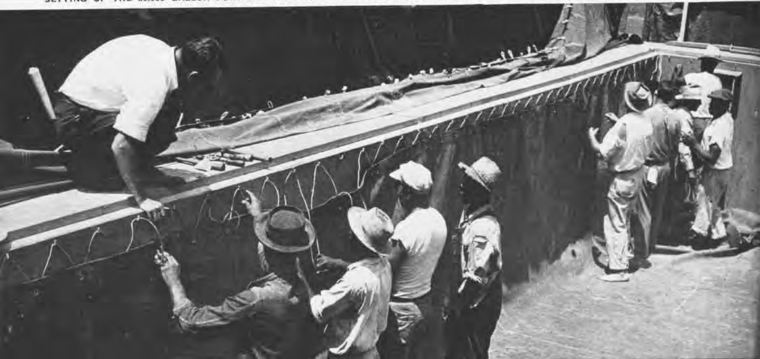
SETTING UP THE 80,000 GALLON PORTABLE POOL IS A THREE-DAY JOB: WORKMEN INSTALL A RUBBER LINER INSIDE THE STEEL TANK
