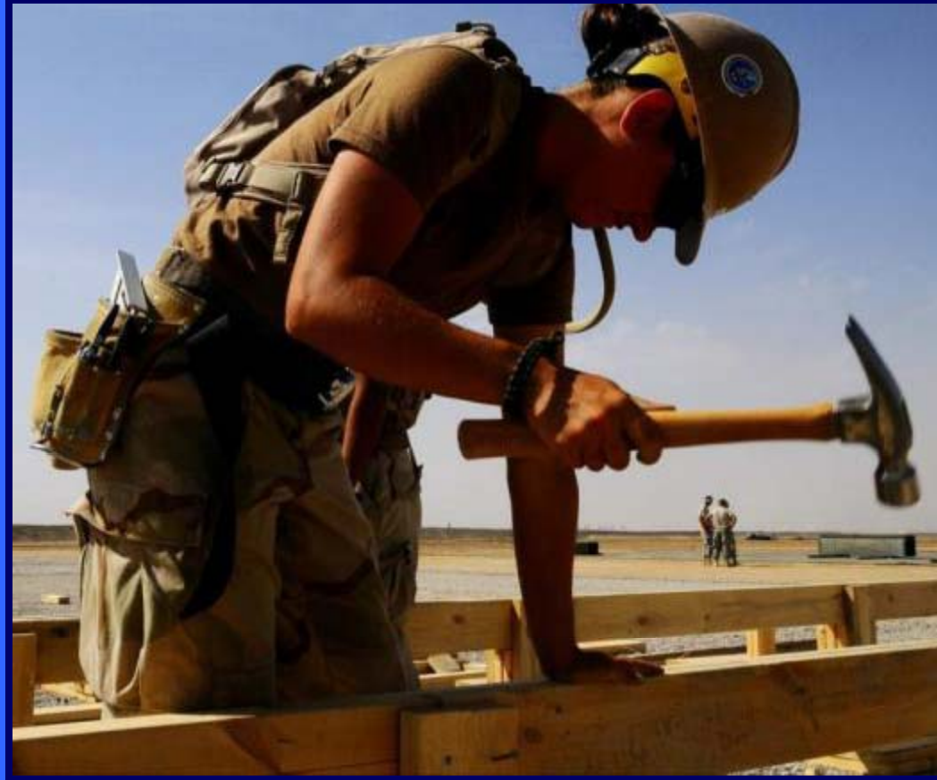
Builder 3rd Class Amy Higgins, a member of the Naval Mobile Construction Battalion 11 Air Detachment in Afghanistan, builds a hut a Kandahar Airfield, 2009.
