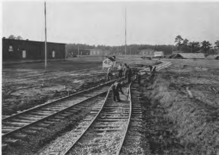
Workers repair railroad tracks at the Naval Ammunition Depot at St. Julien's Creek, Jan. 9, 1939. For many years, this facility manufactured and stored much of the Atlantic Fleet's ammunition. This activity has since been moved up to the Yorktown Naval Weapon Station. Today, St. Julien's is the headquarters of the U.S. Navy's Inactive Fleet and several other Naval activities. (HRNM photo)
