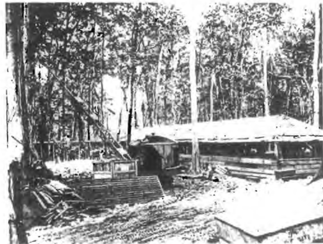
The Chow Hall, First Structure to Go Up in a New Camp
