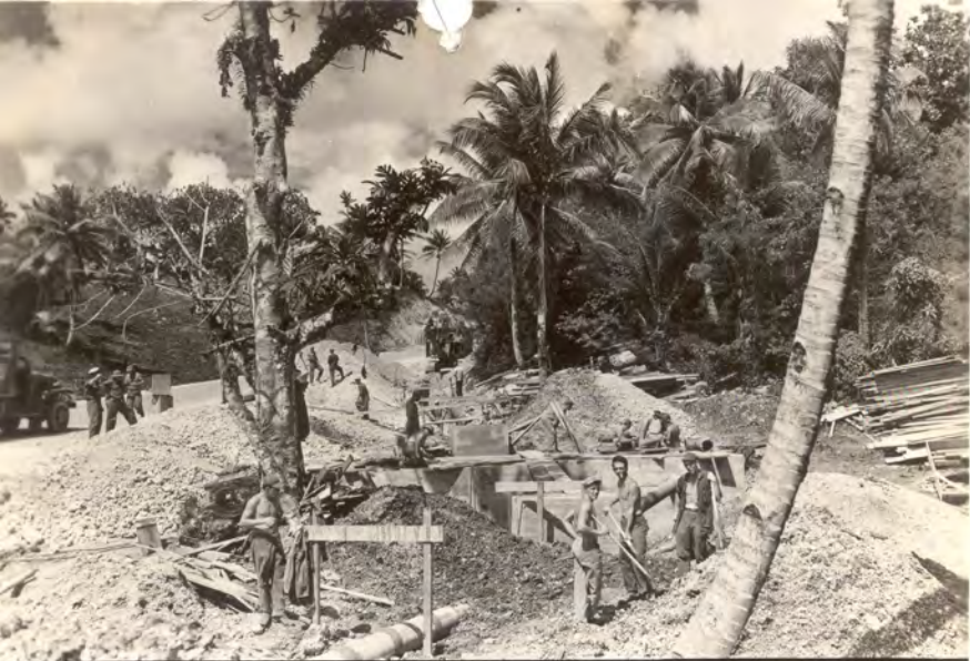
COMPHIBSPAG SEPTIC TANK, CAMP AREA
