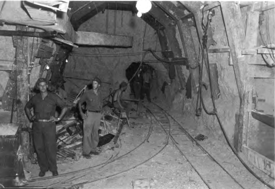
BASAL WATER SUPPLY TUNNEL
