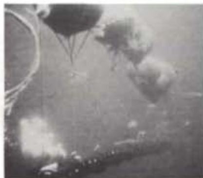
Flotation balloons suspend cable in water while it is being hauled ashore to prevent chafing on the rocky sea floor.
