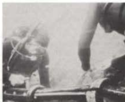
Conventional method of applying split-pipe cable protectors requires divers to install them underwater while cable is still suspended by flotation balloons.
