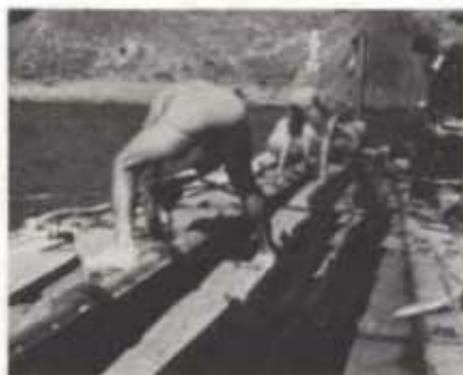
Innovated technique for applying protectors to 30 foot lengths of cable on the beach, after which the length is towed into the water to be submerged and joined with the previously installed sections.
