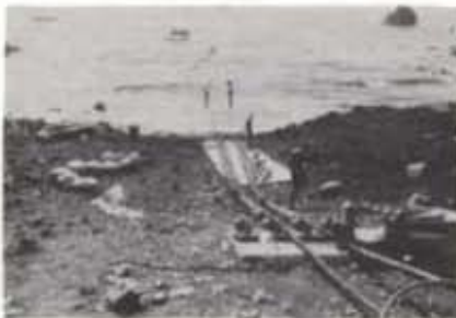
Installing cable protectors in the dry saved nearly one month for the operation as compared with conventional underwater method of installation.
