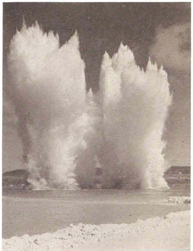
About 3 tons of dynamite was used to blast the sides off reefs less than 60 feet wide
