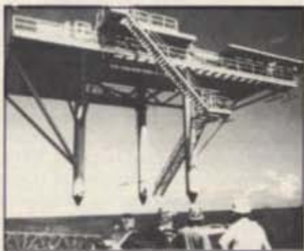
Three hundred-fifty ton deck section of Charleston tactical aircrew combat training system (CTACTS) being lifted for placement.
