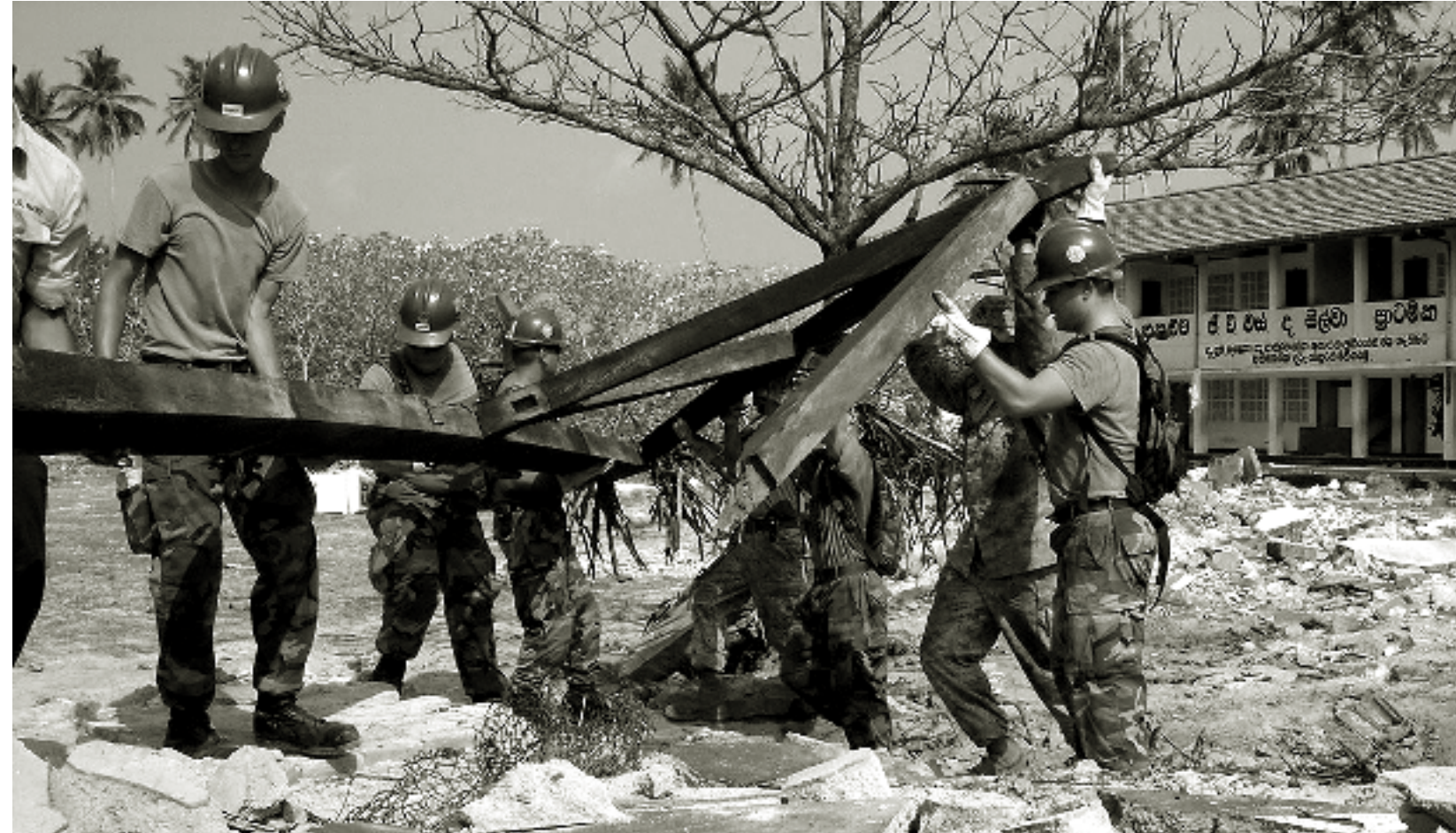
NMCB 7 Seabees, 15th MEU Marines and USS Duluth Sailors remove trusses after a school building is taken down by a Seabee bulldozer.
