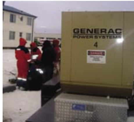
Stand-by generators spool up
