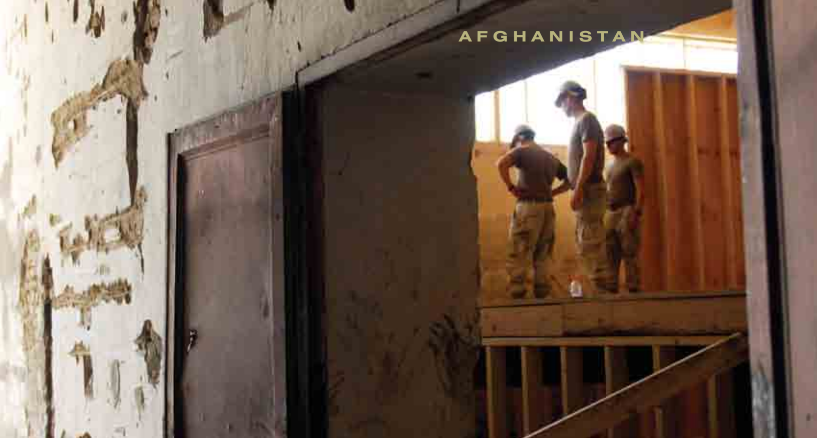
Members of NMCB 133 work on the Tactical Operations Center in the cannery on Camp Nathan Smith, Kandahar City, Afghanistan.
