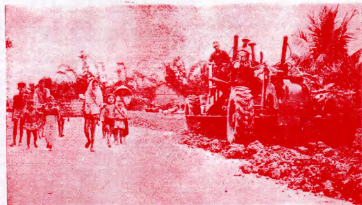
VIETNAMESE TRAINEE is supervised by D. L. Morrison, EO1, of Seabee Team 1007, during construction of the road at Tay Ninh.
