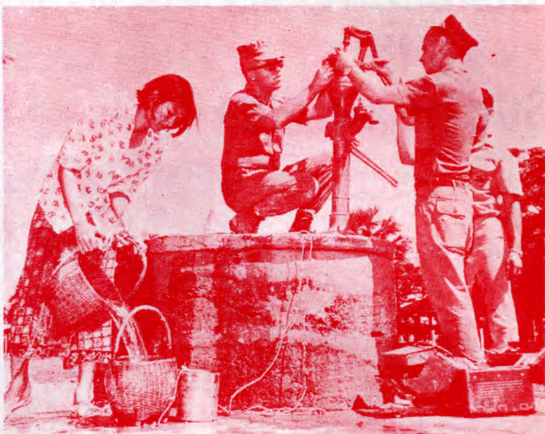
IN THEIR SPARE TIME , Daniel B. Buckley, HM1, and Fred T. Nelson, EAD3, repair a village water pump. The men are with Seabee Team 0306 deployed in Northeastern Thailand, in support of USOM and its accelerated rural development program. Along with Seabee Team 0508, the men are teaching and advising the nationals about the operation and maintenance of construction equipment. The Seabees and their students are building rural roads which give access to villages and small earthen dams which will provide water for thousands of villages during future dry seasons.
