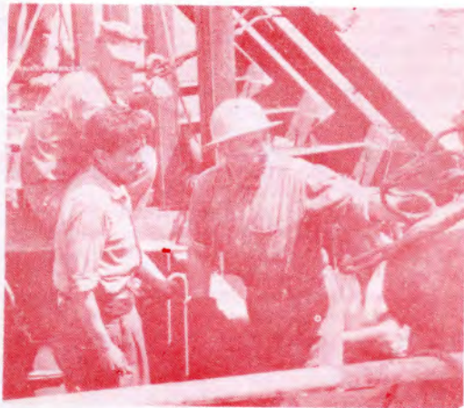
James R. Morton, BUI, USN (center background), and Chilean workers check a form placed on a sheet-pile bulkhead at Talcahuano, Chile.
