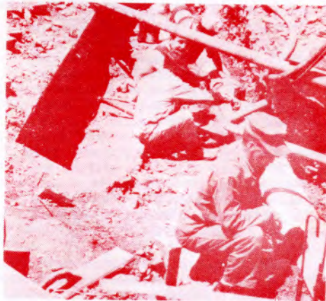
A member of U.S. Atlantic Fleet Seabee Technical Assistance Team (STAT) One supervises Chilean nationals during installation of a drainage line at the Talcahuano, Chile, Naval Shipyard. Wharves at the shipyard were destroyed by an earthquake. U.S. Navy Seabees are providing technical assistance in rebuilding the damaged port area.
