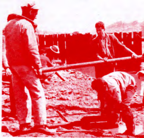
Walter G. Bryzinski, SWI, USN (left), of STAT-1, keeps a watchful eye on the work as Chilean steelworkers install an anchor rod.
