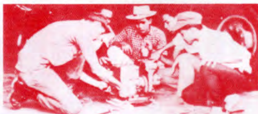
H. Sneed, EOI, USN, instructing Vietnamese trainees in the repair of a water pump.
