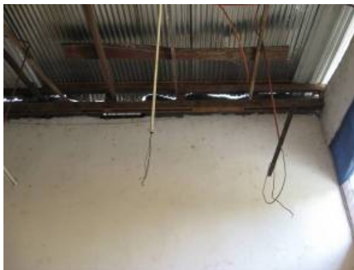
Roof and electrical wiring prior to repair
