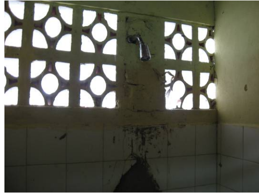
Existing shower fixture
