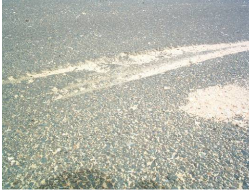
ASR Aspen damage
