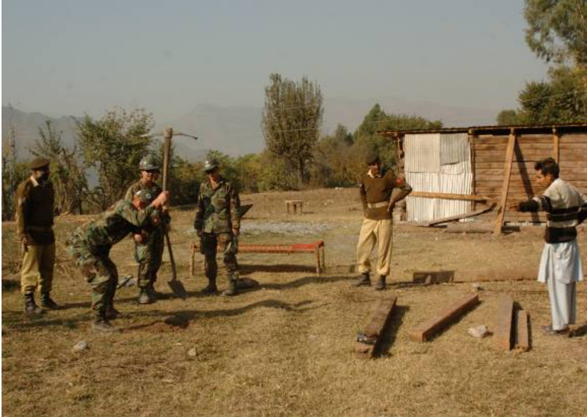
Members of NMCB 74 and Pakistan personnel break ground on a shelter in Miani Bandi Village as the future resident helps direct the work.
