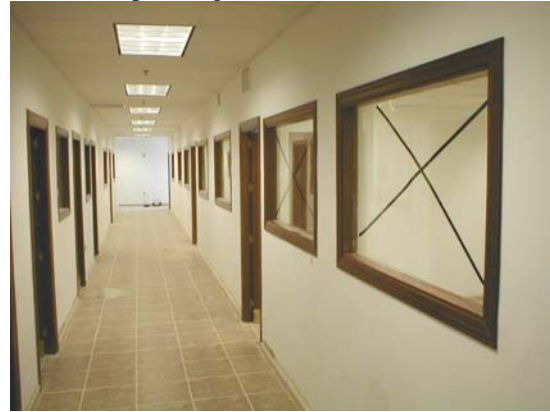
LEFT: Project at turnover. BOTTOM: Main hallway with installation of floor tile and drop ceiling.
