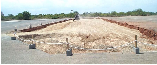
LEFT: Excavated section of parking apron BOTTOM: Completed section of parking apron being put to use
