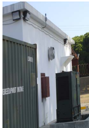
Wall Pack Lighting
