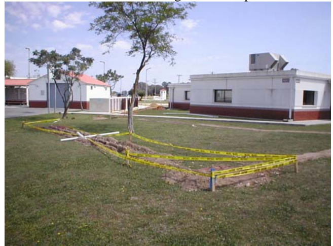
LEFT: Ball valve and solenoid valve to connect to existing sprinkler system BOTTOM: 3” main line running around hospital.
