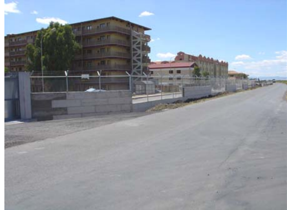
LEFT: Wall west of Galley Gate in February. BOTTOM: Section six of wall west of gate.
