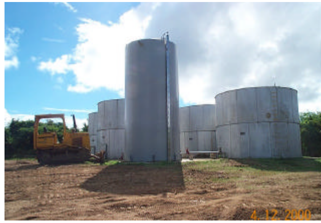
Completed new water tank
