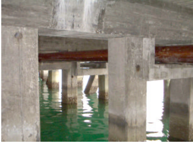
Fire Protection Pipes under pier had to be replaced
