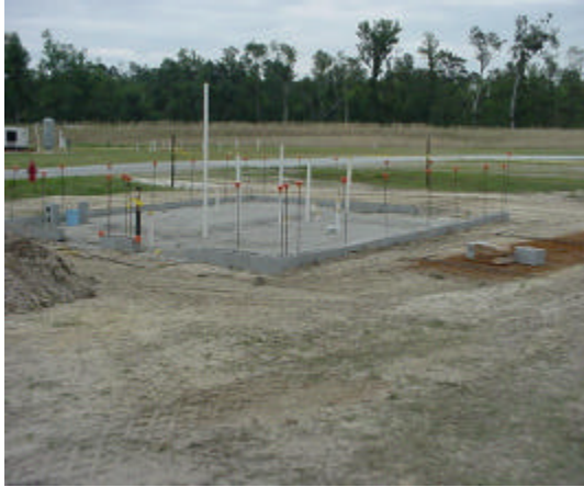
Footings, slab, underslab plumbing, and the first course of block in place
