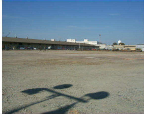
Parking area has been cleared and grubbed. Ready to install parking bumpers at Deans Hardwoods (Phase II)
