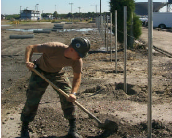
Crewmember installing security fence for parking area at South Gate (Phase I)
