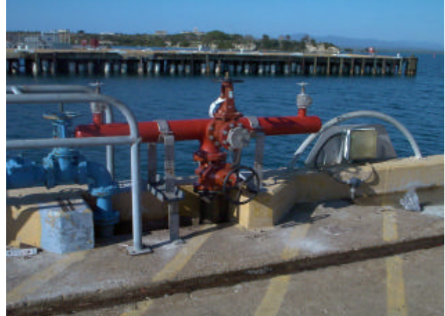
New Fire Suppression section
