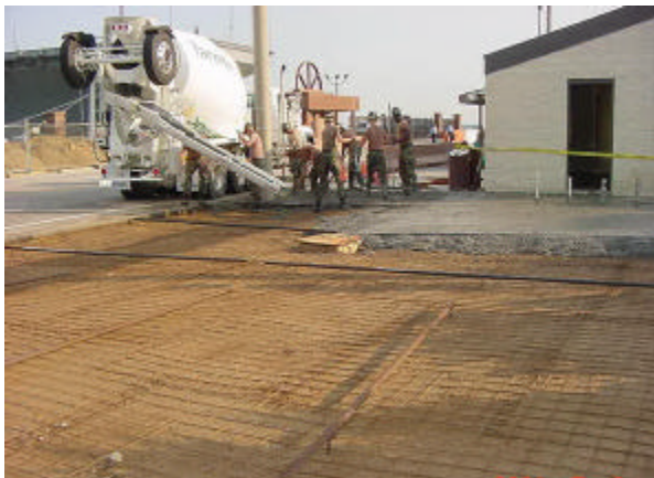
Placing concrete at pier 12 Naval Station Norfolk for the Atlantic Fleet phone bank
