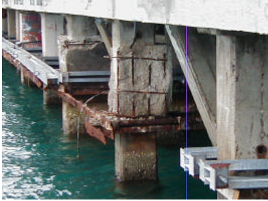
Above: Failed Concrete Piles Right: Fender Sections being installed
