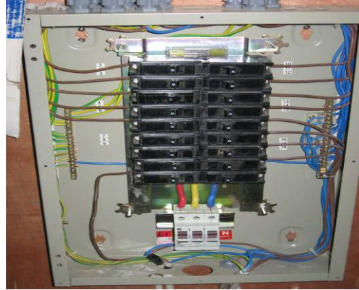
New sub panel
