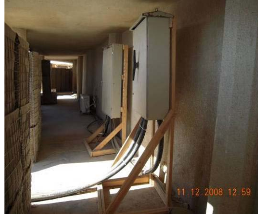
New MDP and transfer switch
