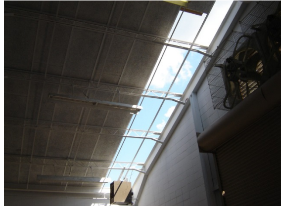
An inside view of the facility where the roof panels have been blown off.
