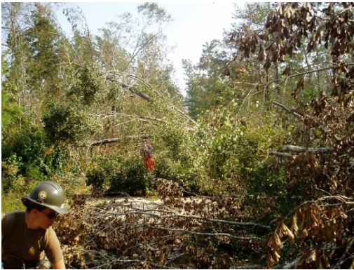
Road crew sawing and removing fallen trees from roadways
