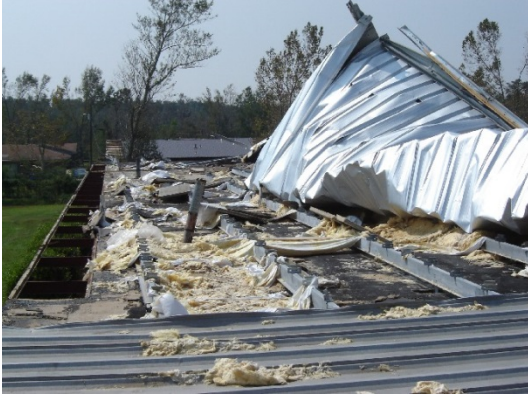
Extent of damage to roof at Lucedale Intermediate School
