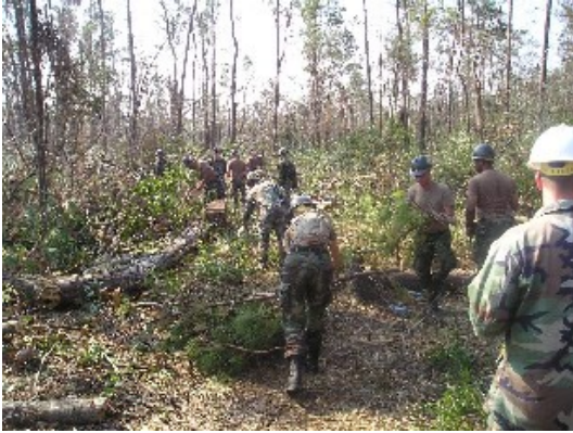
Seabees from NMCB-7 clear land to create a stable foundation for future construction.
