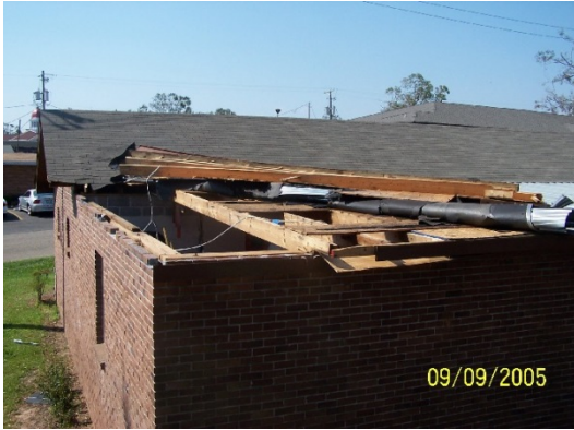
Damage to the facility.
