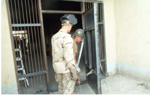
Left: Two NMCB SEVEN steelworkers repair a door at the prison in Ad Diwaniyah.
