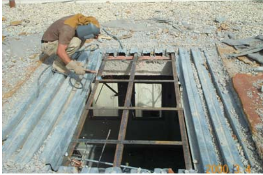
Left: A Seabee welds the support structure for a patch over the arty hole.
