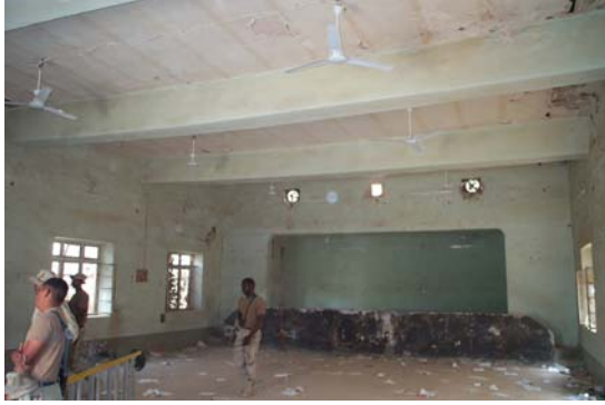
Left: NMCB SEVEN personnel survey the Al Markazia school for damage.
