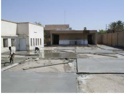
Left and Below: Iraqi laborers tore out the courtyard and replaced the tile and concrete.
