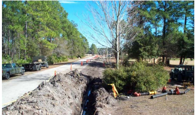
Left: Excavating to place new water line. Bottom: Backfilled and landscaped section of new water line.
