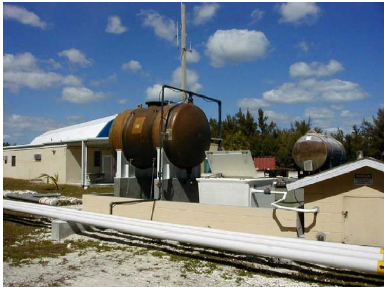
Left: Pump and hose reel (April 2001). Below: Tank, separator and containment sump (April 2001).
