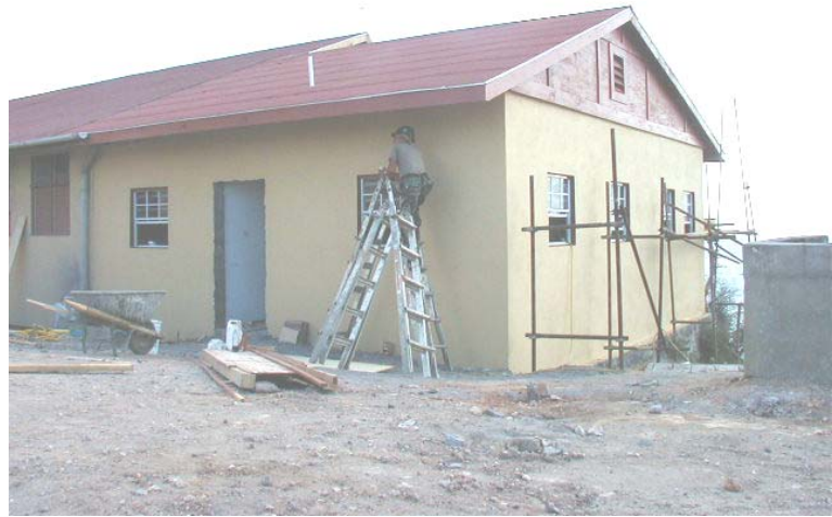
Left: Initial site preparation for footer. Below: Putting the finishing touches on the clinic.
