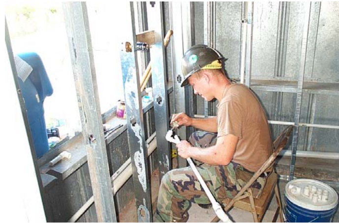
Seabees started from scratch to renovate berthing buildings. Left: Finishing sheetrock. Below: Installing plumbing.
