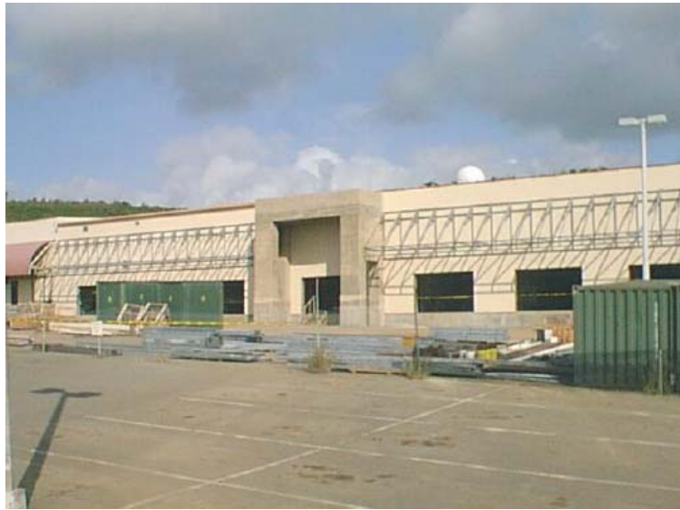
Left: Concrete slab and columns (October 2000). Below: Current view of expansion (May 2001).
