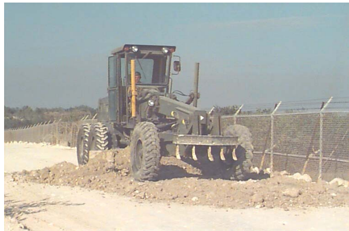
Left: Applying the first of two layers of aggregate for DBST. Below: Raising the road elevation to desired height.
