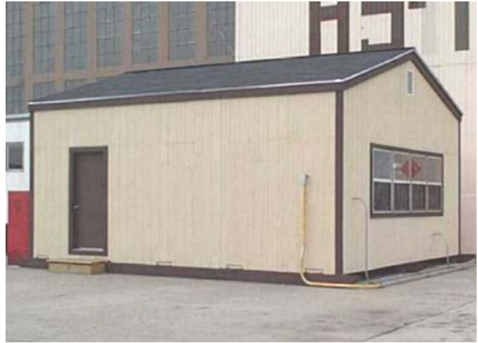
Left: The rough framing of building number one. Below: Completed building (December 2000).
