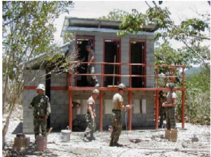
Left: The toilets were formed and poured with concrete. Below: Completed latrine.
