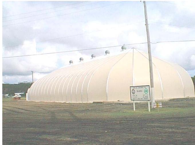
Left: The crew erecting the tension fabric structure. Below: The completed structure (March 2000).
