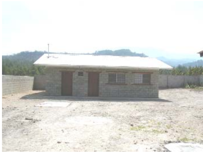
Left: EOCA Green rolls the site in preparation for placing concrete pad (February 2001). Below: Completed medical clinic (April 2001).
