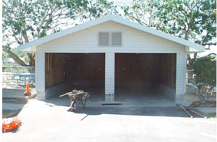
Left: Inspecting the existing slabs. Below: Carport 1 during the final phases of construction.
