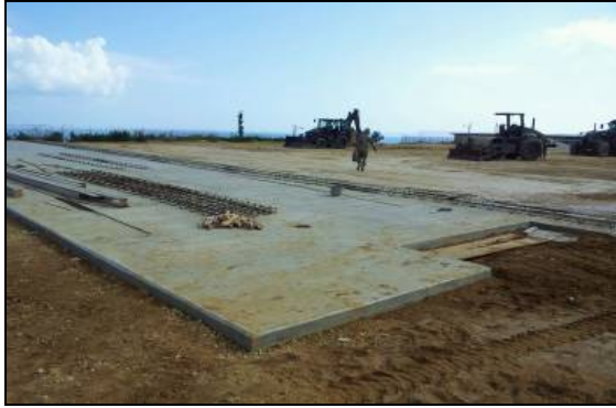
At left, the beginning of Communication Pad A. Below is the completion of Communication Pad C.
