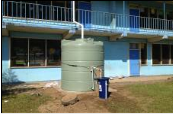
Water catchment systems installed at Apia Primary School and Samoa College.
