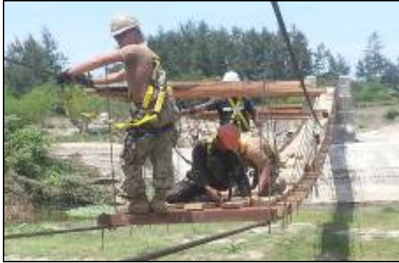
At left, Seabees from NMCB 5 install decking for the footbridge. Below, the completed footbridge pictured from the west side of the river.
