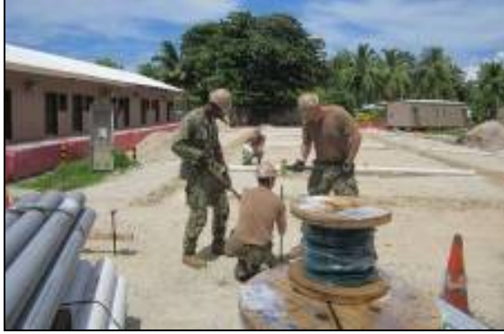
At left, Seabees from NMCB 5 work to prepare the initial site. Below, the completed facility as it nears turnover with NMCB 3.
