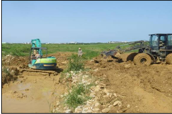
At left, Seabees from NMCB 5 perform excavation of project site. Below, site before suspension of work
