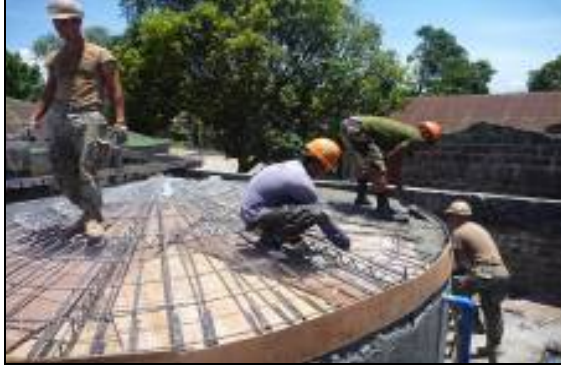
At left, the partnered crew applies stucco to the roof. Below, the completed water tank pictured.
