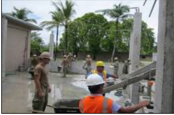
At left, Seabees from NMCB 5 corefill the first six courses of the CMU wall. Below, the completed facility as it nears BOD.
