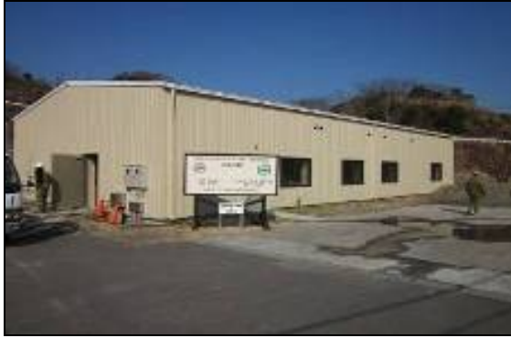
At left, the initial site conditions are pictured. Below is the interior in late June 2013.
