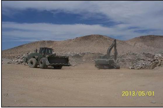
At left, Seabees from NMCB 5 work to prepare the initial site. Below, ¾” minus aggregate is loaded into a dump.
