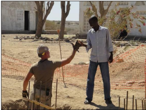
SW1 (SCW) Johnson high fives one of the locals, while digging trenches for Kontali Clinic grade beams
