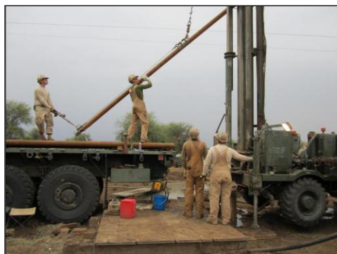
Seabees install pipe for the water well rig in Dire Dawa, Ethiopia
