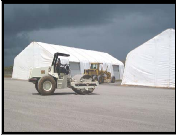
Gravel at tension fabric warehouse.
