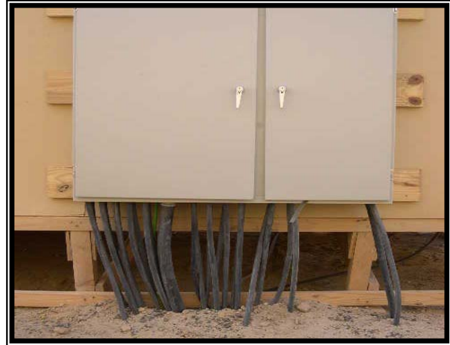
Completed electrical panel.
