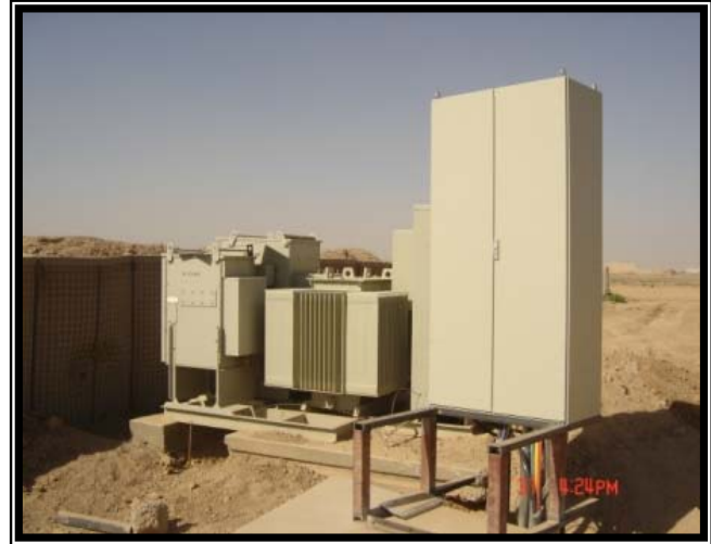
Completed transformer and panel box.
