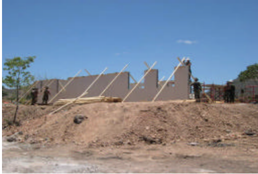
Seabees from NMCB 5 erect the Royal Building System walls for the two-room schoolhouse.
