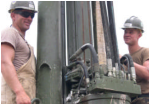
EO1 Jensen and CM3 Hudson make repairs to the rig's top head motor
