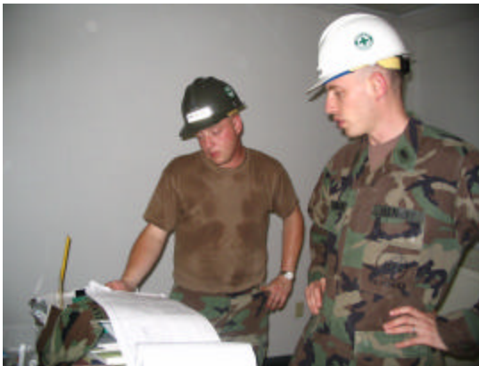
Medical-Dental Clinic Renovation crew leader and Medical Officer confer over clinic architectural plans
