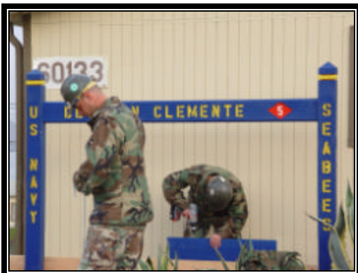
Construct Detail OIC/ AOIC Sign.
