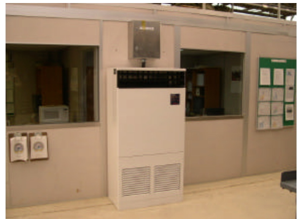
Heater installed in work area of TFS.
