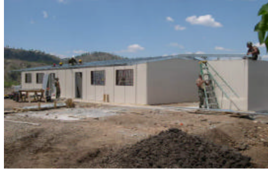
The USARSO designed roof is being installed on the school and head.
