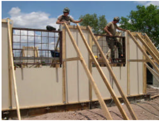
CECN Krnichar and BU3 Young run a string line during a QA inspection.
