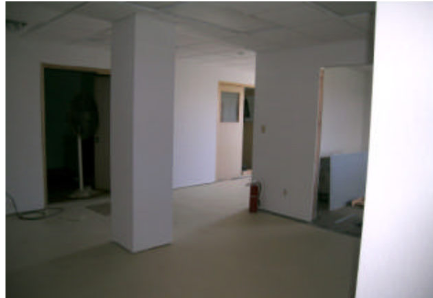
At left, Seabees installing drywall metal studs. Below, renovated sections shown at turnover with NMCB-133.
