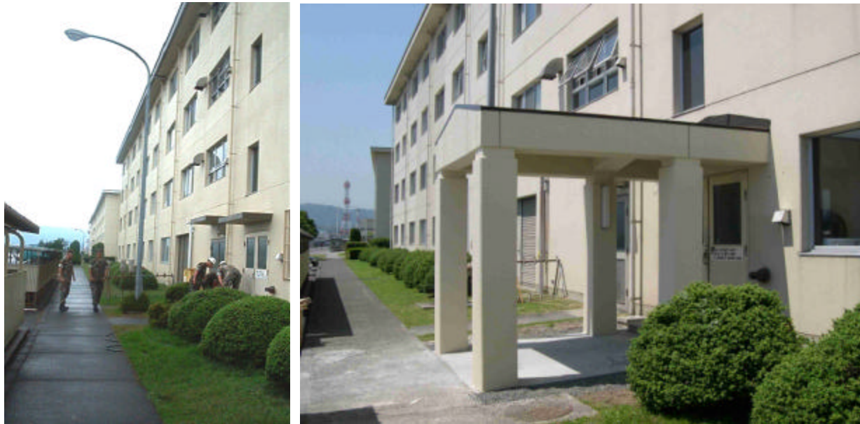
At left, original rear canopy of bldg 314 prior to construction. Right, completed canopy with new walkway and roofing.
