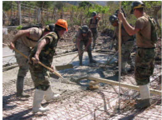
The Sitio Viejo crew work hard to place the concrete pad for the school, using a pump trailer and 3” pipe.
