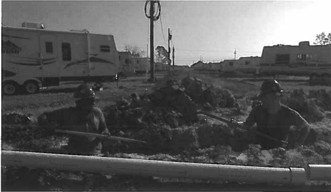
050928-N-2653P-067 Plaquemines Parish (Sept 28, 2005) - Utilitiesman Gregory Knight and Hospital Corpsman 1st Class Joshua Ross assigned to Naval Mobile Construction Battalion Four Zero (NMCB-40), dig trenches for sewage lines for 19 trailers for evacuee families. The Navy's involvement in the Hurricane Katrina humanitarian assistance operations are led by the Federal Emergency management Agency (FEMA), in conjunction with the Department of Defense. U.S. Navy photo by Journalist 1st Class James Pinsky (RELEASED)
