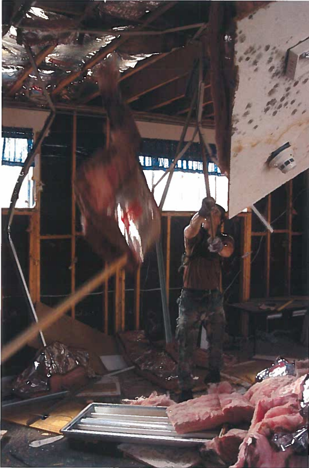
050922-N-9712C-005 New Orleans (Sept. 22, 2005) - U.S. Navy Equipment Operator 3rd Class Slade Miller, assigned to Naval Mobile Construction Battalion Four Zero (NMCB-40), removes water damaged insulation from the ceiling at Saint Rosalie School in New Orleans. The Navy's involvement in the
