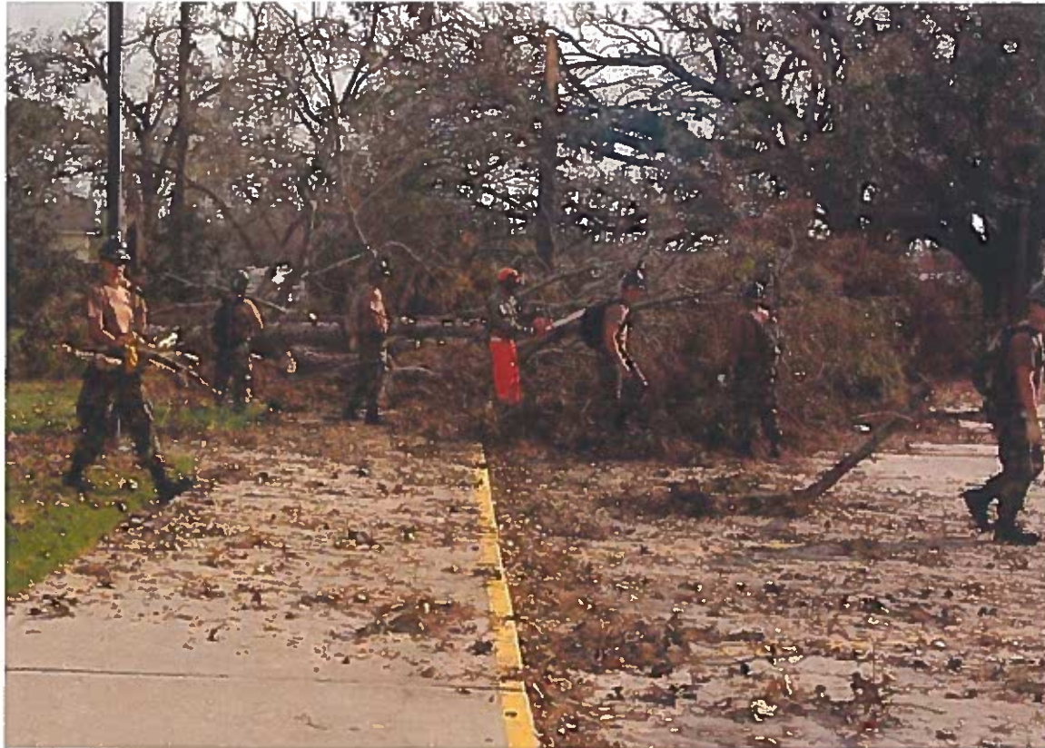
050912-N-9274T-006 New Orleans (Sept. 12, 2005) - Seabees assigned to Naval Mobile Construction Battalion Four Zero (NMCB 40) out of Port HUENEME Calif., clears away debris around the Plaquemine Parish Post Office in Louisiana in support of Hurricane Katrina relief efforts. The Navy's involvement in the Hurricane Katrina humanitarian assistance operations are led by the Federal Emergency Management Agency (FEMA), in conjunction with the Department of Defense. U.S. Navy photo by Photographer's Mate 2nd Class William Townsend (RELEASED)
