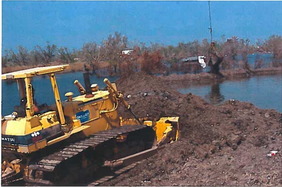
050915-N-9712C-002 Buras, La. (Sept. 15, 2005) - U.S. Navy Equipment Operator 1st Class Max Lopez, assigned to Naval Mobile Construction Battalion Four Zero (NMCB-40), uses a bulldozer to supply a crane with loose dirt to block the area where Buras Levee broke during Hurricane Katrina. The Navy's involvement in the Hurricane Katrina humanitarian assistance operations are led by the Federal Emergency Management Agency (FEMA), in conjunction with the Department of Defense. U.S. Navy photo by Photographer's Mate 3rd Class John P. Curtis (RELEASED)
