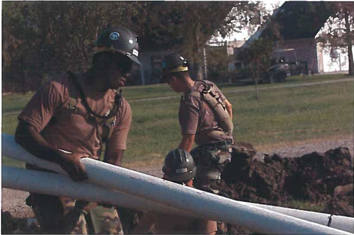
050928-N-2653P-007 Plaquemines Parish (Sept. 28, 2005) - Seabees from Naval Mobile Construction Battalion Four Zero (NMCB-40) prepare to install sewage pipes for an evacuee relocation trailer site. The land, donated by a local Plaquemines Parish resident, will house 19 families and will have full water, electrical and sewage facilities. The Navy's involvement in the Hurricane Katrina humanitarian assistance operations are led by the Federal Emergency management Agency (FEMA), in conjunction with the Department of Defense. U.S. Navy photo by Journalist 1st Class James Pinsky (RELEASED)
