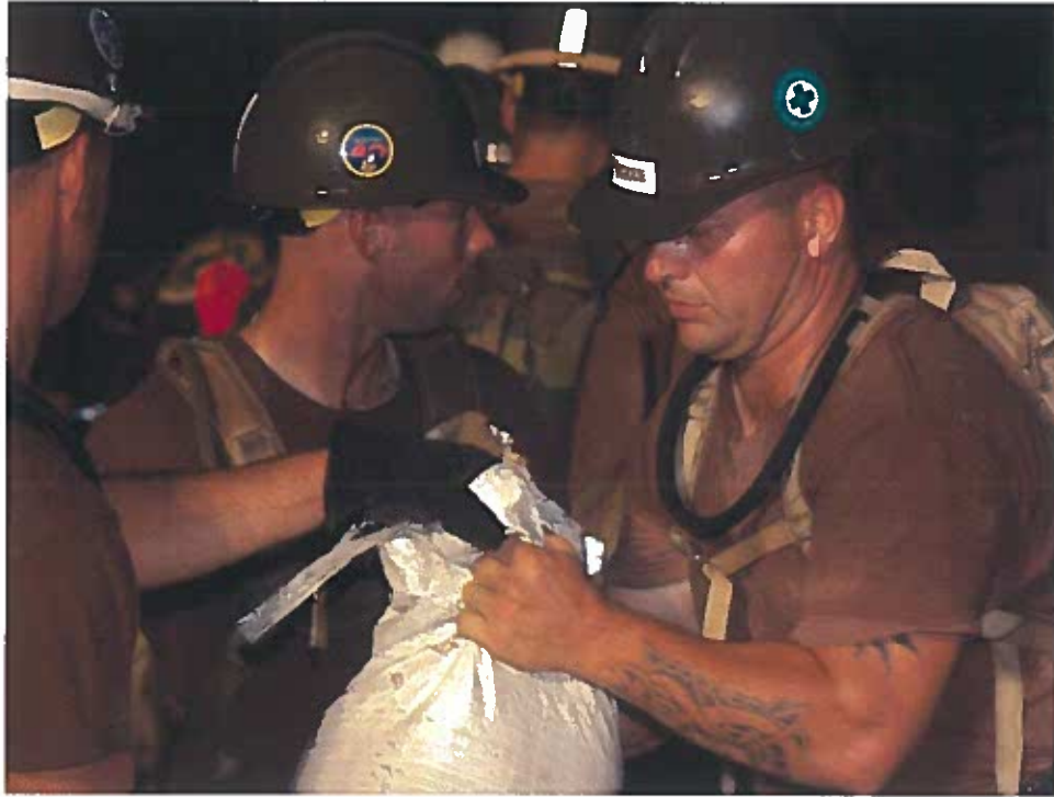
050924-N-0000X-001 New Orleans (Sept. 24, 2005) - U.S. Navy Builder 1st Class Daniel McKee (right), assigned to Naval Mobile Construction Unit Four Zero (NMCB-40), hands-off a sandbag to another Seabee while repairing a levee. The Navy's involvement in the Hurricane Rita humanitarian assistance operations are led by the Federal Emergency Management Agency (FEMA), in conjunction with the Department of Defense. U.S. Navy photo (RELEASED)
