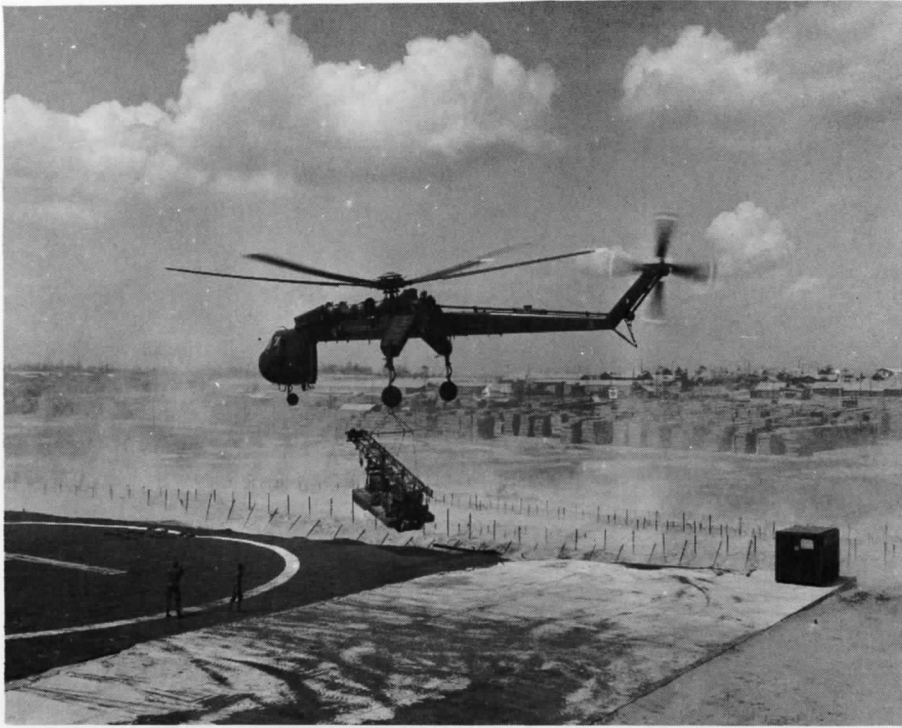
A SEABEE first - The well rig was disassembled and the pieces flown to Thoung Duc. The crew then reassembled the rig and drilled the well
