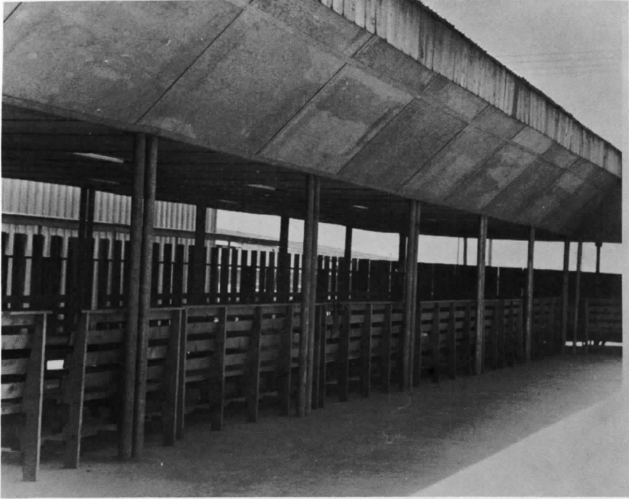
A project dear to the heart of SEABEES and MARINES was the reconstruction of the Freedom Hill Beer Garden
