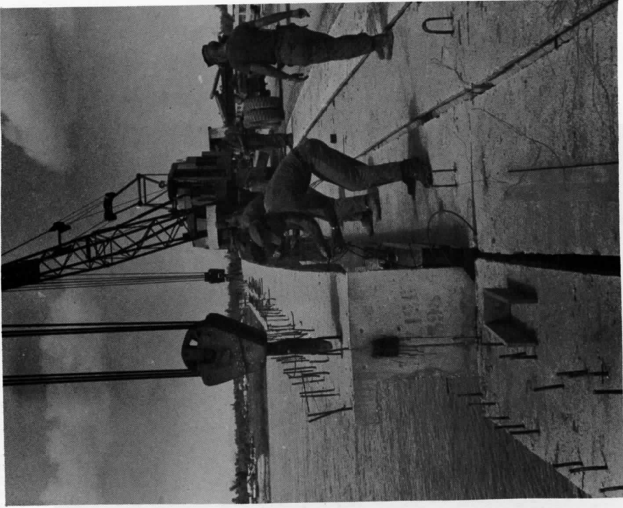
Cau Lau Bridge-Threading post tensioning cables as the last edge beam is lowered into place
