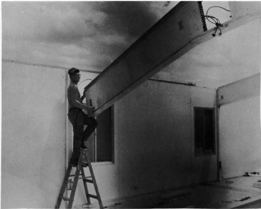
The relocatable Lewis building at Naval Hospital was easily erected without special lifting gear
