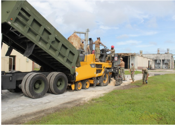
Detail Guam Seabees and 554th RHS practice sand laydown in preparation for upcoming paving evolution
