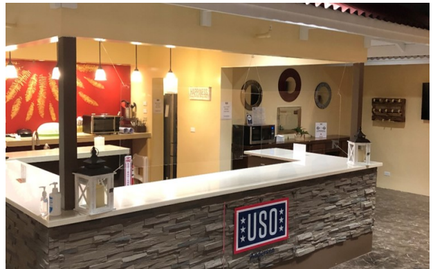
Installed sneeze guard at USO.
