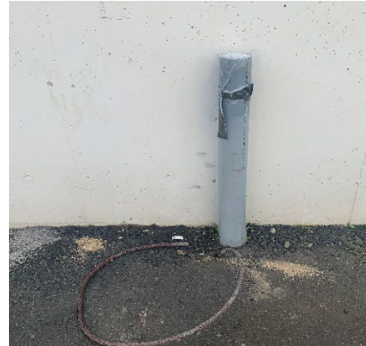
4 inch Plumbing PVC Used as Electrical Conduit
