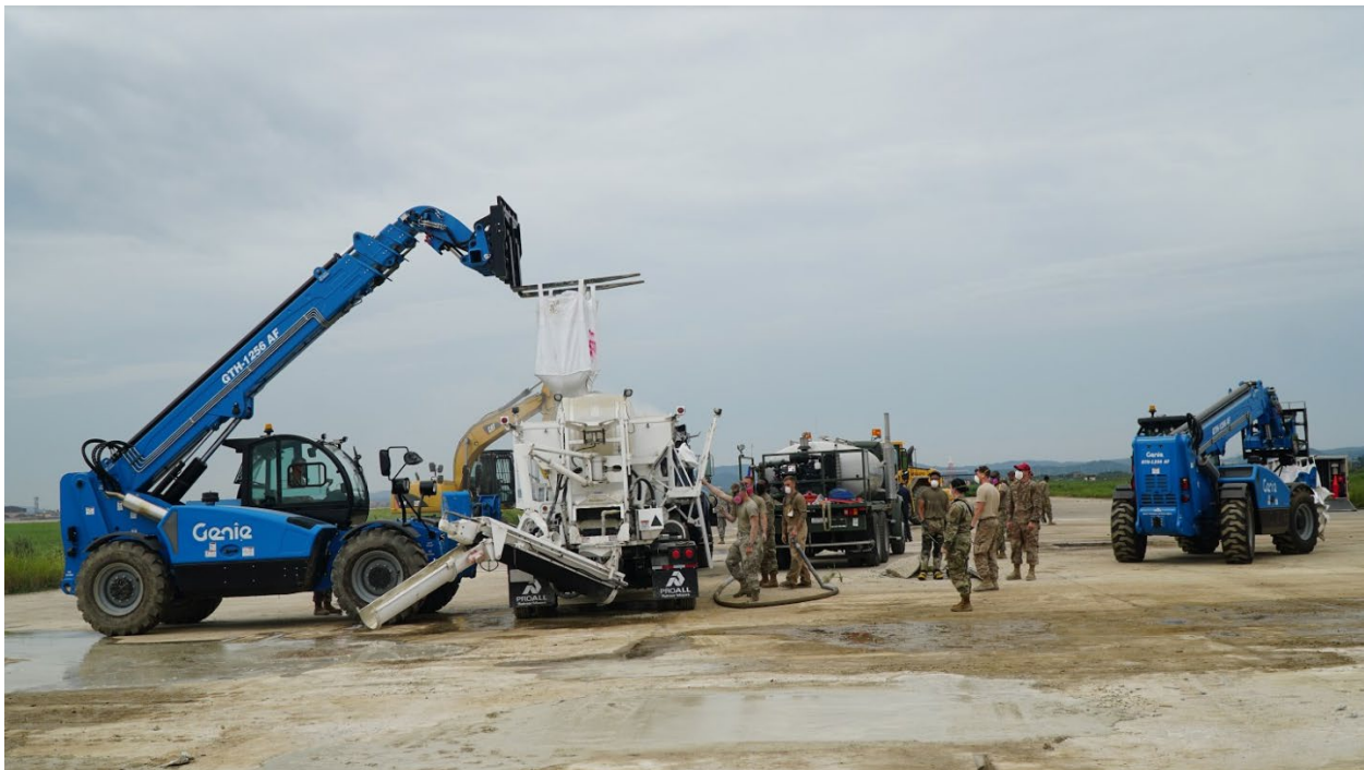
Seabees and USAF personnel work together to repair a runway during Silver Flag Exercise.
