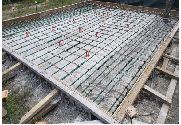
Installed RST and forwork in preparation for baler pad concrete pad placement.
