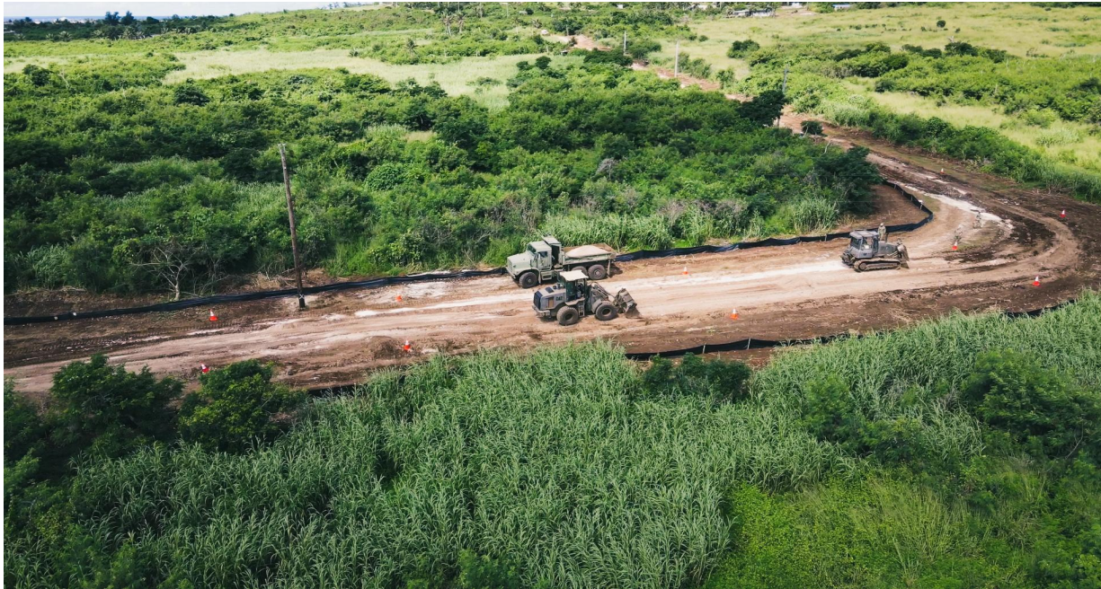
Detail Tinian Seabees perform excavations in support of Marpo Heights Road G
