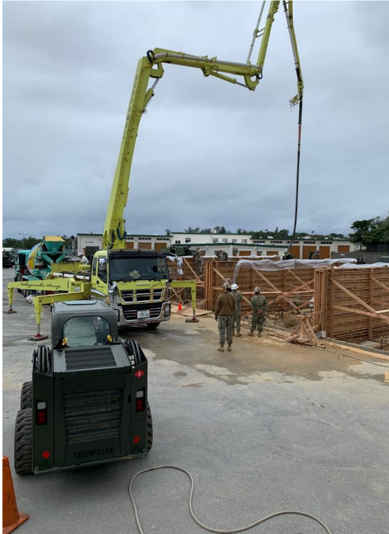
Seabees conduct overhead concrete placement for four 9 ft concrete walls for CESE wash rack on Camp Shields.
