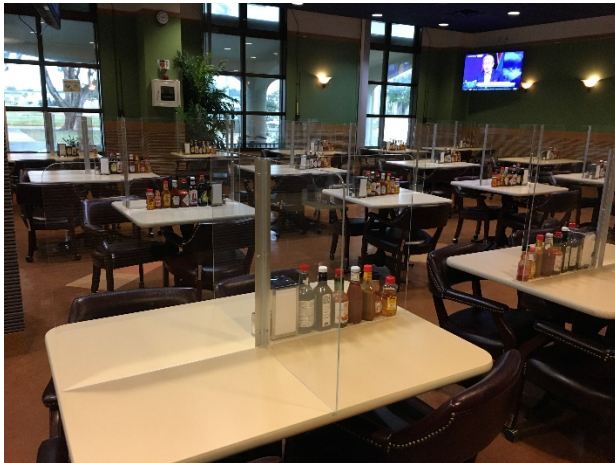
NMCB THREE Seabees installed COVID mitigation barriers on galley tables allowing Camp Shields galley return to dine-in services.
