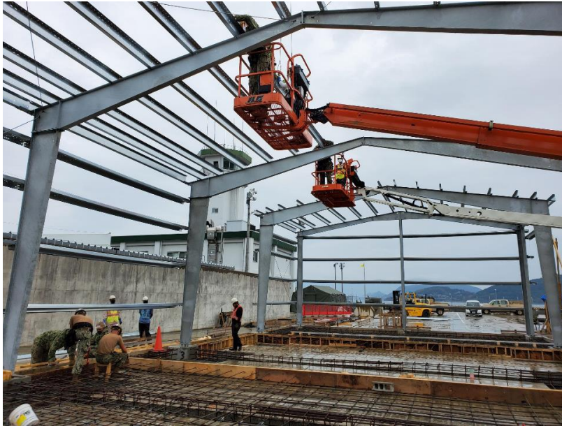
Seabees and Public Works Department Sasebo crane crew install purlins for one of two PEBs being constructed for NBU 7.
