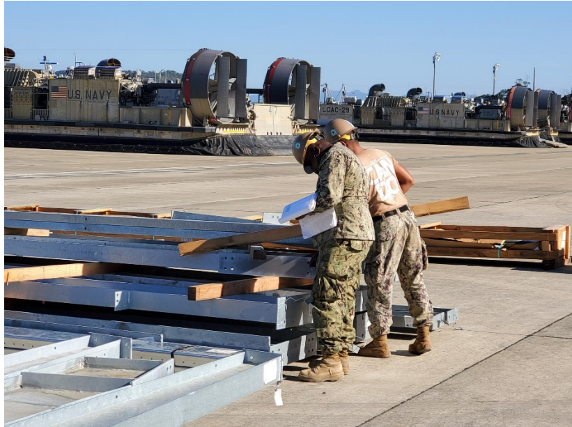
Seabees organize structural steel members of the PEB. The two PEBs will support NBU 7 LCAC (in background) maintenance and operations.
