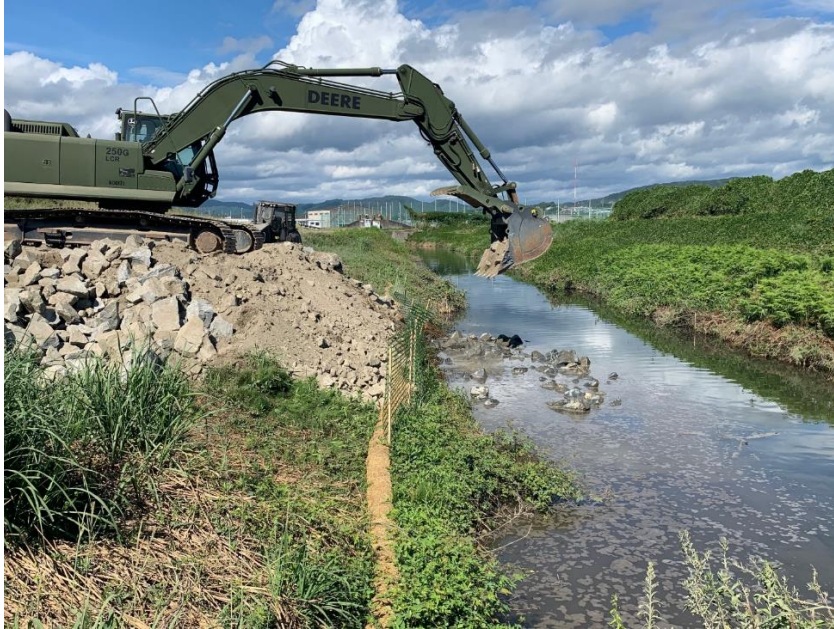
Seabees conduct joint operations with MWSS 172 constructing a 30 ft culvert bridge for the landfill cap project.
