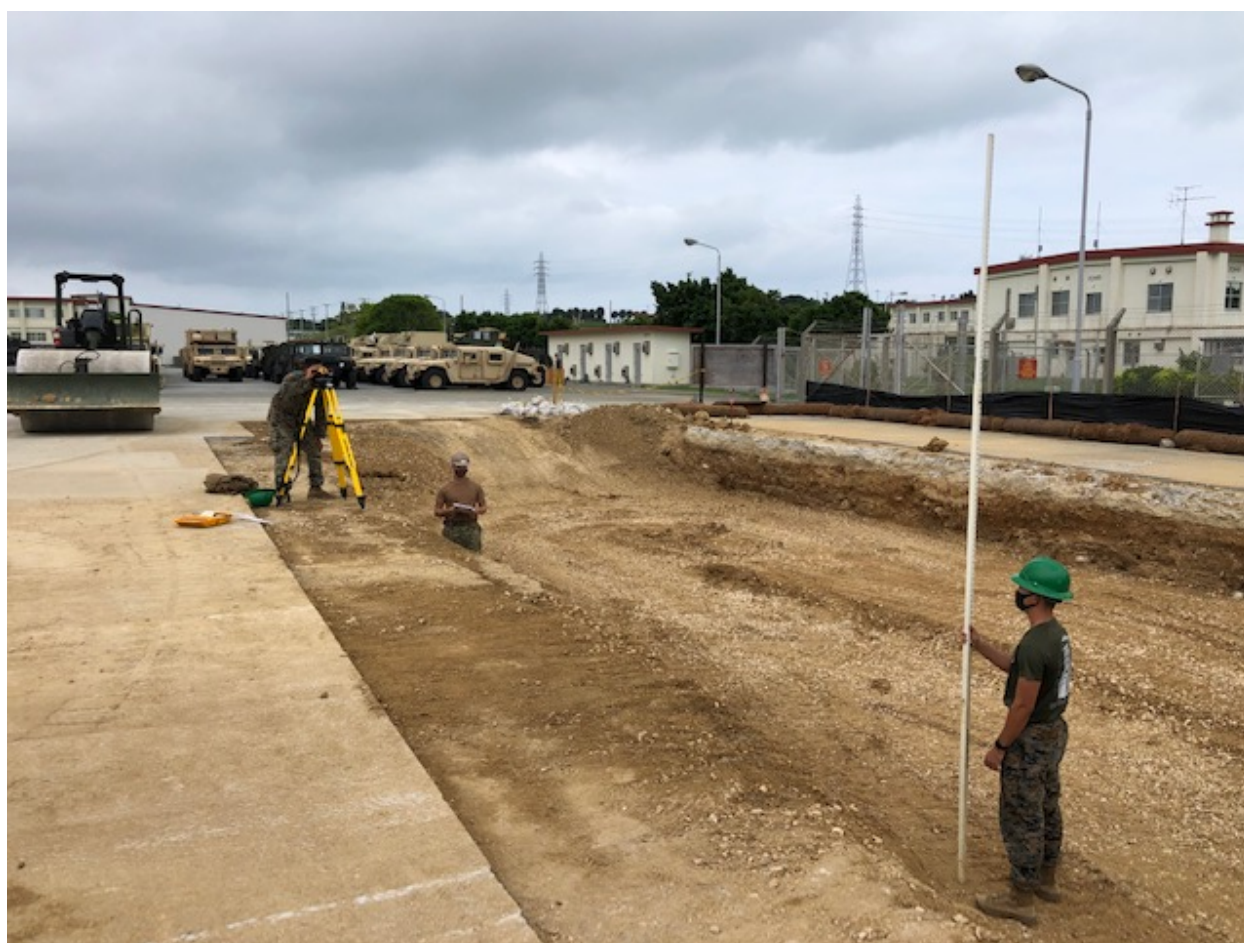
NMCB THREE Engineering Aides and 9 th ESB Marines measure the progress of backfilling the 5 ft deep excavation site at JK18-877 G/ATOR Support Facilities project.
