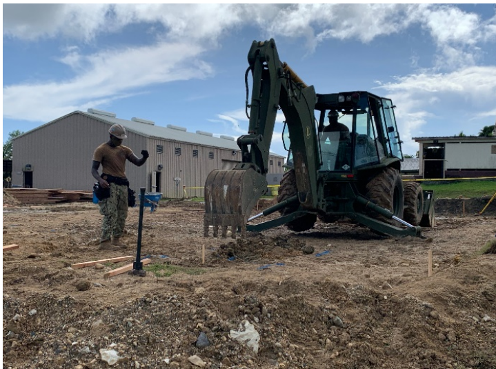
Detail Palau Seabees excavate and remove spoils in support of a CLU facility on Camp Katuu
