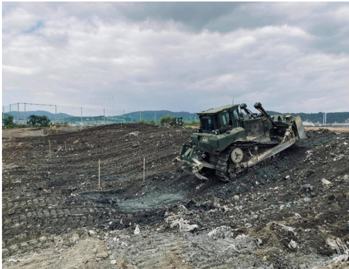
Seabees and 9 th ESB Marines conduct earthwork operations for the Marine Corps Air Station Iwakuni landfill project.
