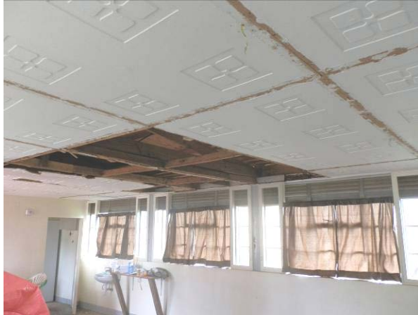
Galley before repair
