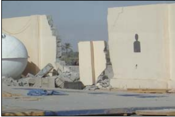
Damaged perimeter wall
