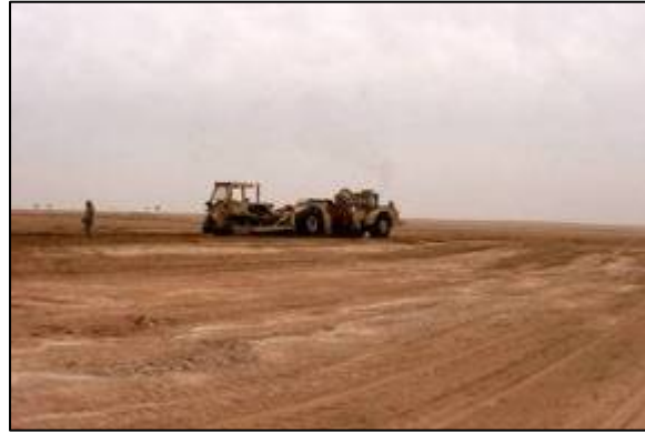
Improved rain water basin
