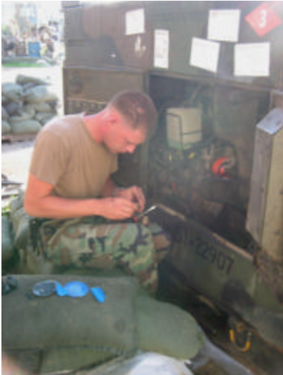
CM's and CE's alike spent many hours maintaining and repairing our three generators that provided power 24/7 for 5 months.
