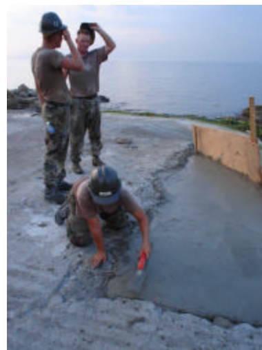
Widening existing boat ramp at Sangley Point for safety and to accommodate larger boats for SEAL Teams
