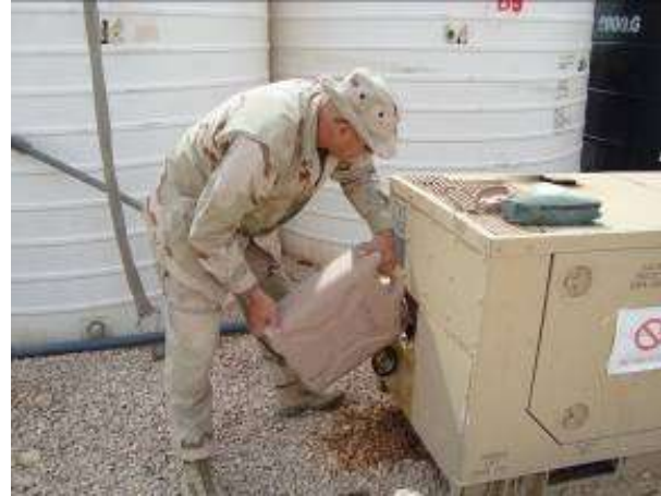
Seabee refills diesel generator
