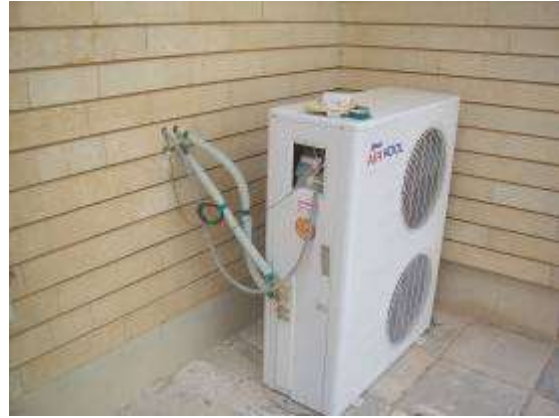
AC Condenser installed
