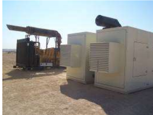
New generator installed
