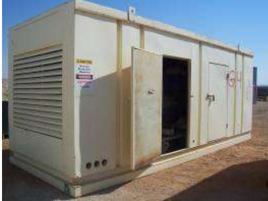
New Generator to be prepped
