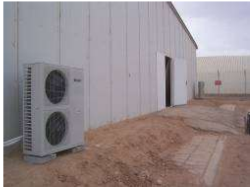
Concrete loading pad and A/C installed
