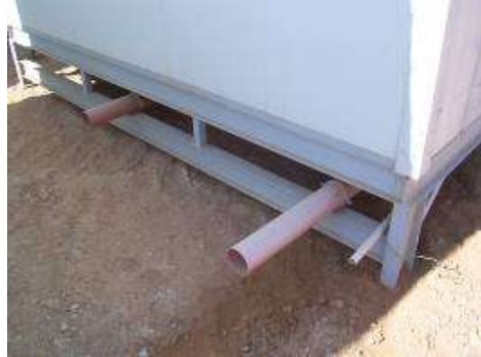
Piping installed at AB Unit
