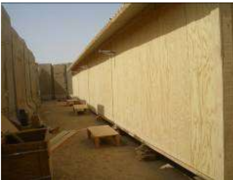
HVAC rough-in and stands
