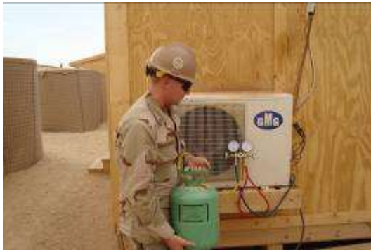
Recharge is provided to HVAC
