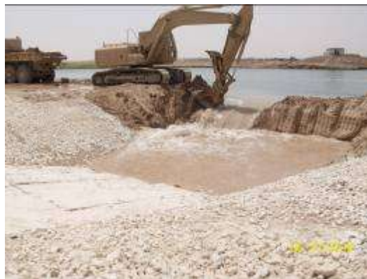
Excavator breaks levy at ramp
