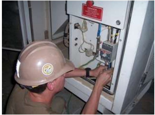
A properly-sized breaker is installed
