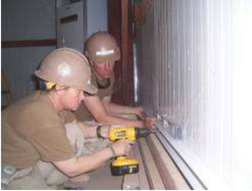
Electrical Raceway installed
