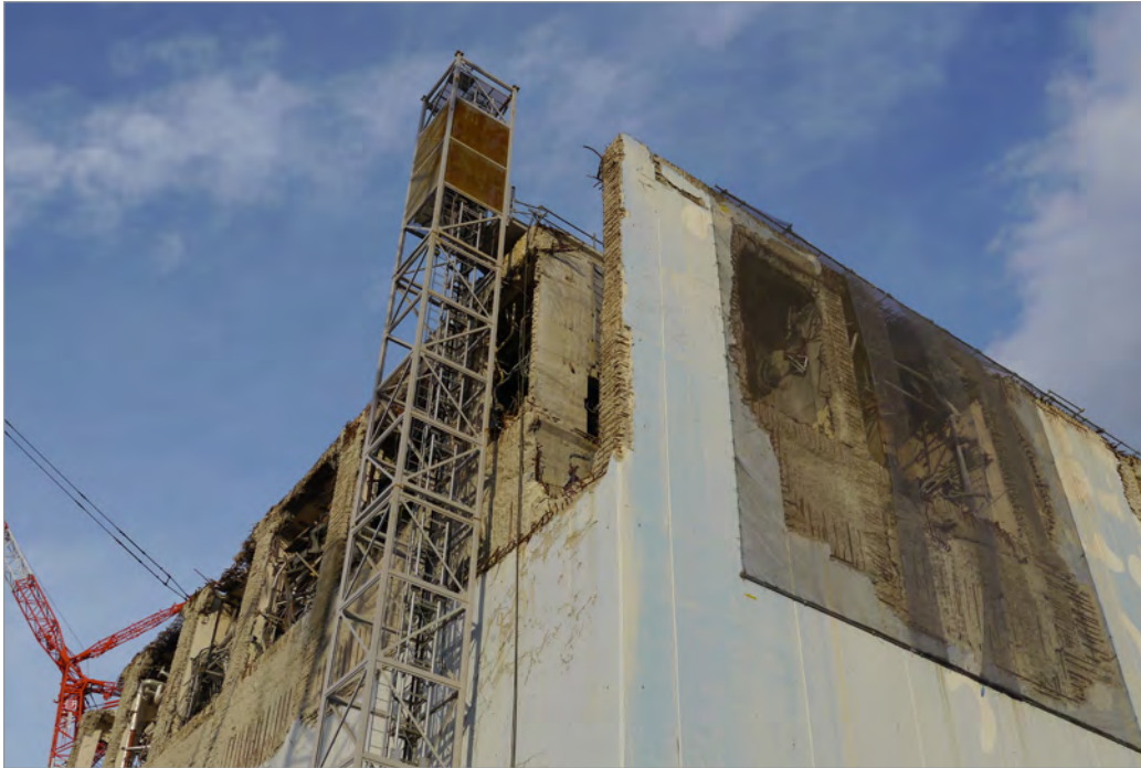
The remains of the building housing Unit 4 after hydrogen explosions there on 15 and 16 March 2011. This photo was taken on 18 December 2021. (Gill Tudor, IAEA; Unit 4 IAEA Photo)
