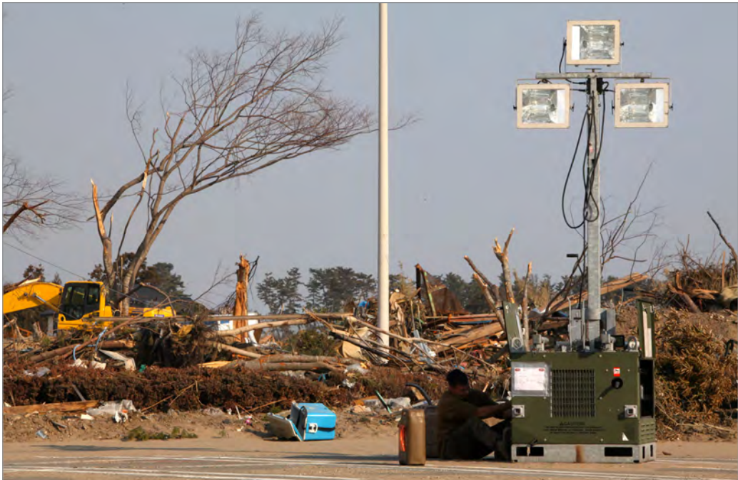
Lance Corporal Robert Branch, an electrician attached to the 3rd Marine Logistics Group, repairs a generator-powered floodlight at the Sendai airport on 29 March 2011. (Gunnery Sgt. J. L. Wright Jr., USMC; DVIDS, 383924)
