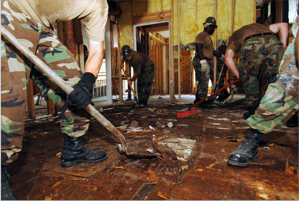
U.S. Navy Seabees assigned to Naval Mobile Construction Battalion 133 (NMCB-133) remove plywood sub-flooring in order to restore Hope Haven, a shelter for abused and neglected children, in Waveland, Mississippi, during Katrina relief operations. (NARA, DN-SD-06-03698)
