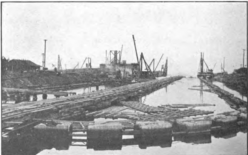
Dry Dock No. 1, Naval Station, Pearl Harbor, Hawaii. General view during construction, showing sections in place.
