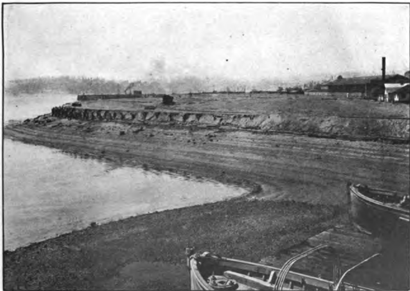
Filling operation in progress, Navy Yard, Puget Sound, Wash., showing extension of shore line.
