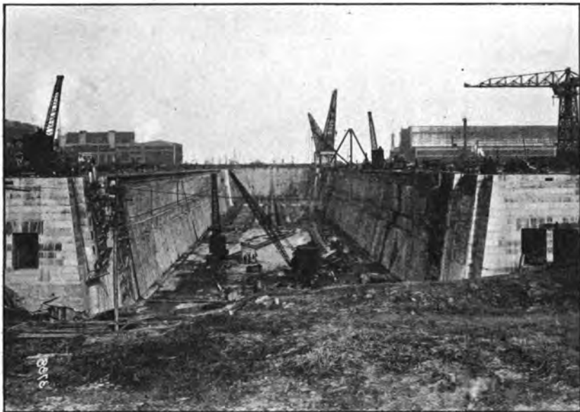
Dry Dock No. 3, Navy Yard, Philadelphia, Pa., under construction. View taken from cofferdam at entrance.
