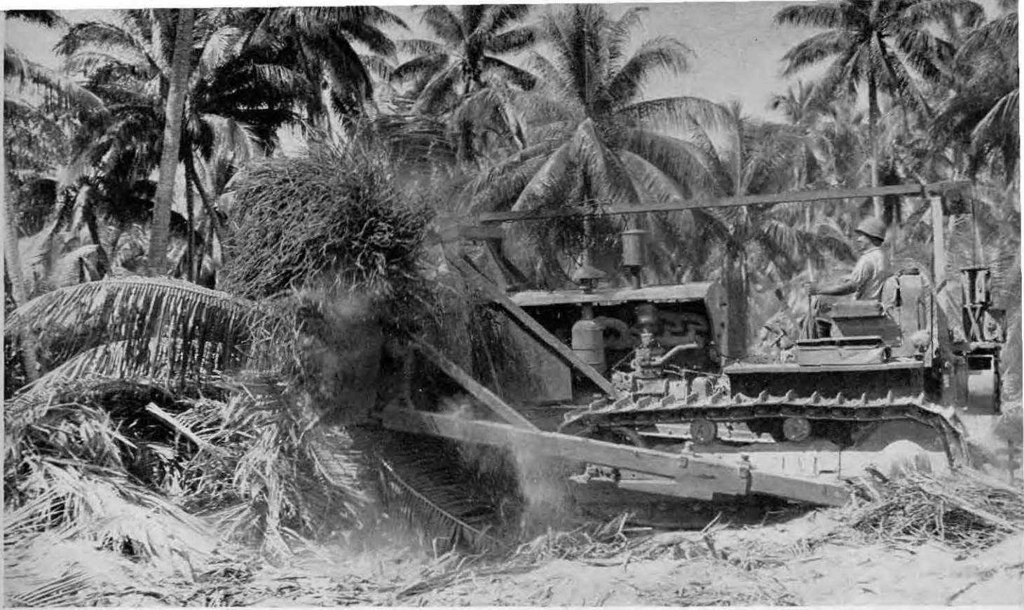
Preliminary clearing and grubbing operations at center of runway; December 5, 1943. Operator C. K. Jones.
