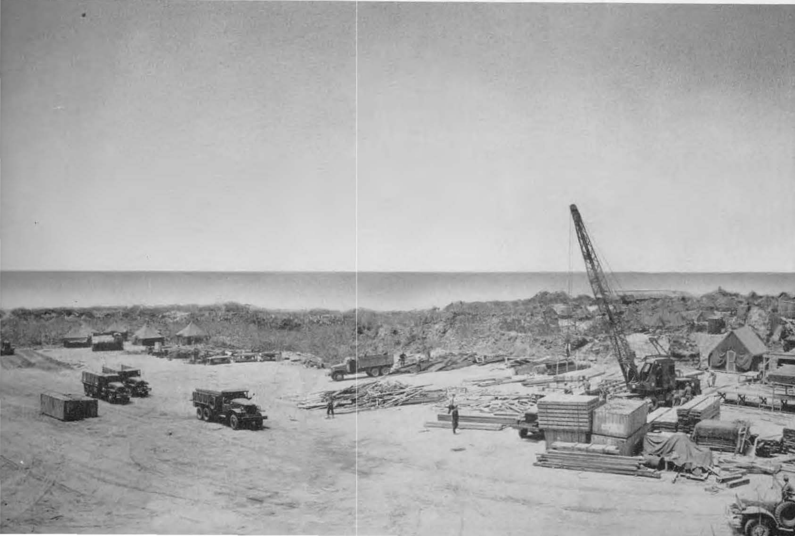
Lead out in the background of center sections. Chow Hall in center. Lumber yard and Carpenter shop at extreme right.
