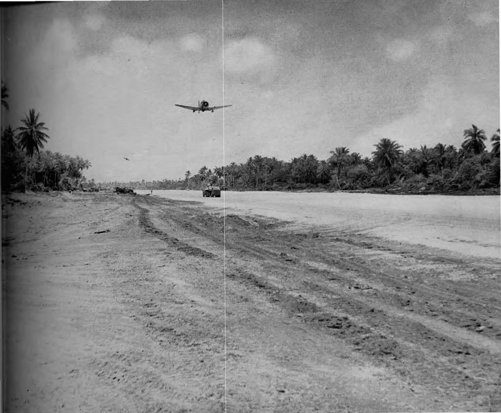
Partially graded but not completely surfaced, the new O'Hare Field was ready December 10, 1943; the first plane is pictured, ready to land December 13, 1943.
