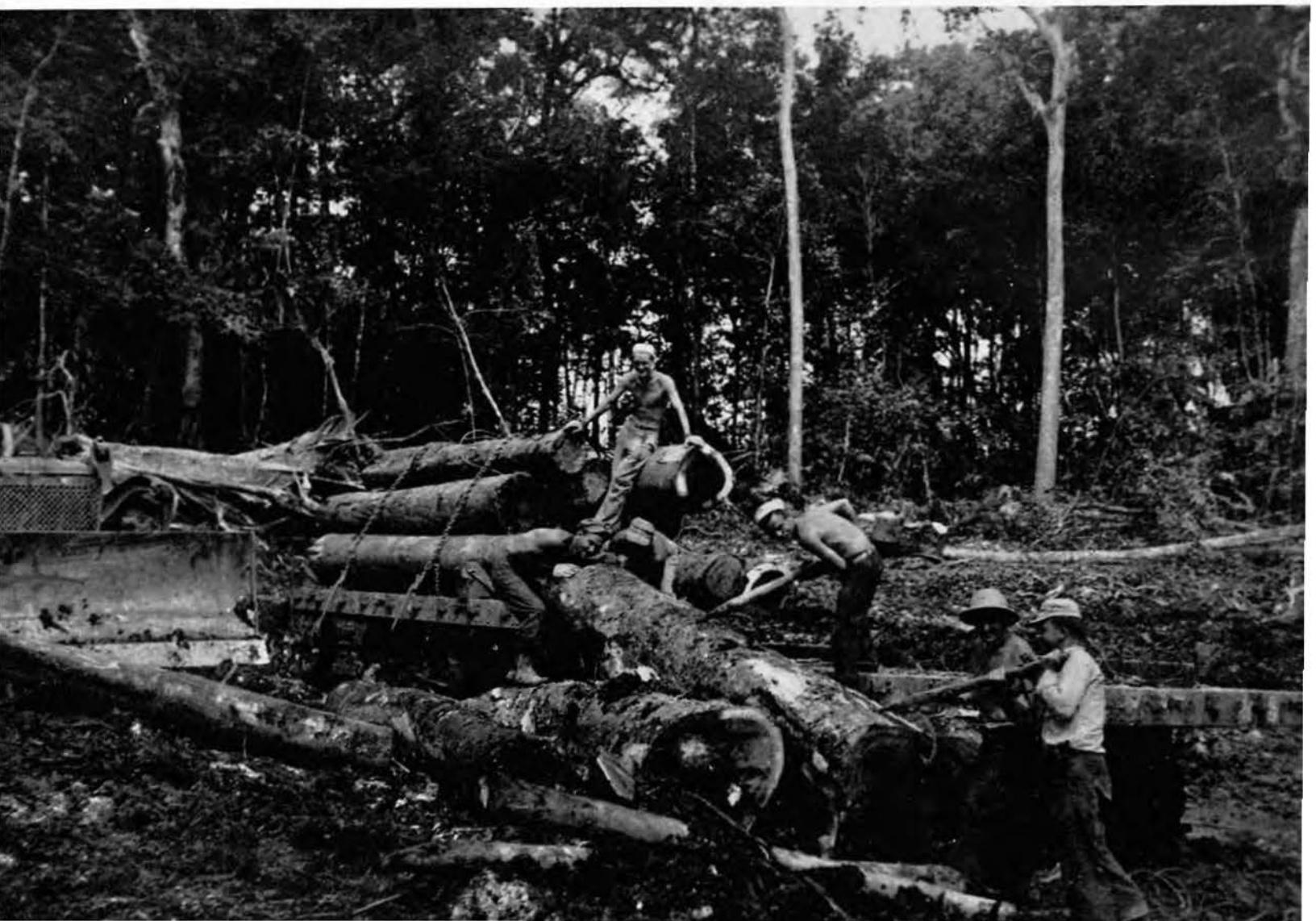
TAXIWAYS HAD TO BE FINISHED WITHOUT DELAY. HARDWOODS TEAKWOOD, MAHOGANY, AND EBONY TREES LEFT DEEP ROOTS EMBEDDED INTO THE CORAL. . . SEABEES APPLIED THE BULLDOZER, LOGGING CREW, AND DYNAMITE AND SOON HAD THE JOB ON THE WAY
