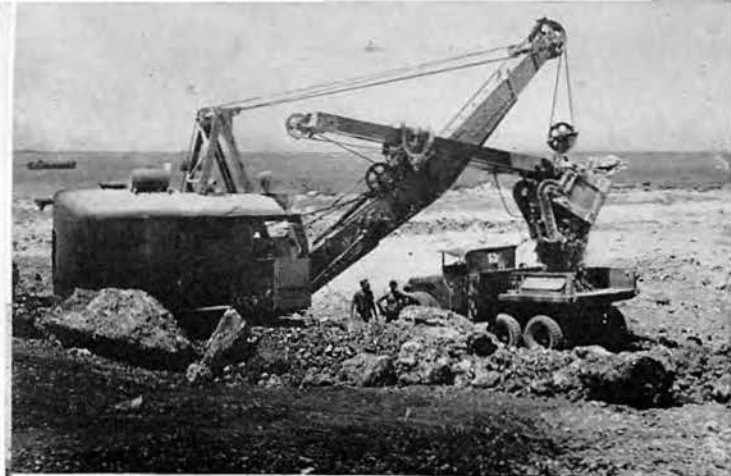
THE SHOVELS AND TRUCKS ARE KEPT BUSY BRINGING CORAL TO THE AIRFIELD
