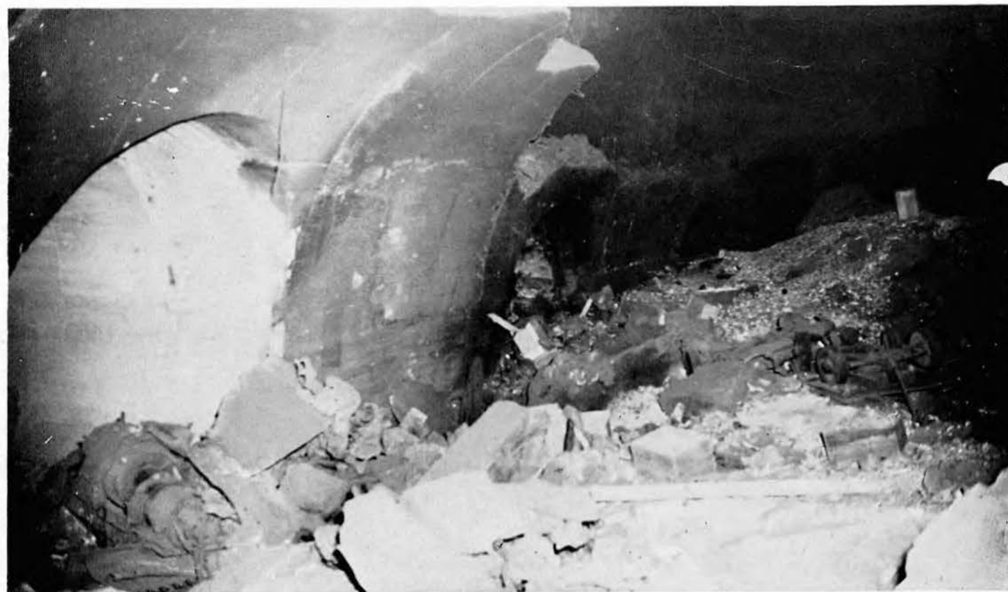
Rubble In Wainwright Tunnel
