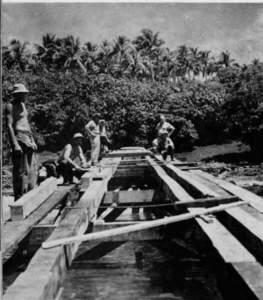
Heavy timbers are laid by Seabees of the 7th Battalion to form the superstructure of a bridge.
