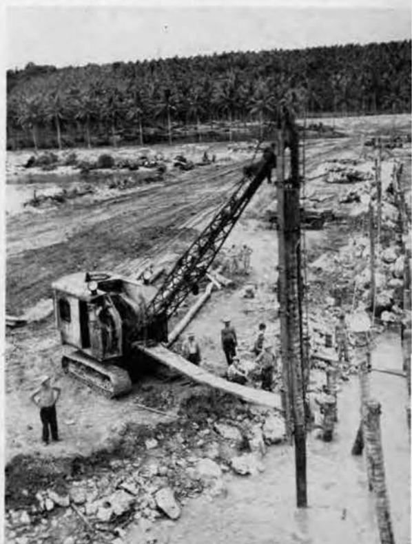
The piledriver does a bang-up job at protecting a road fill from water-wash.
