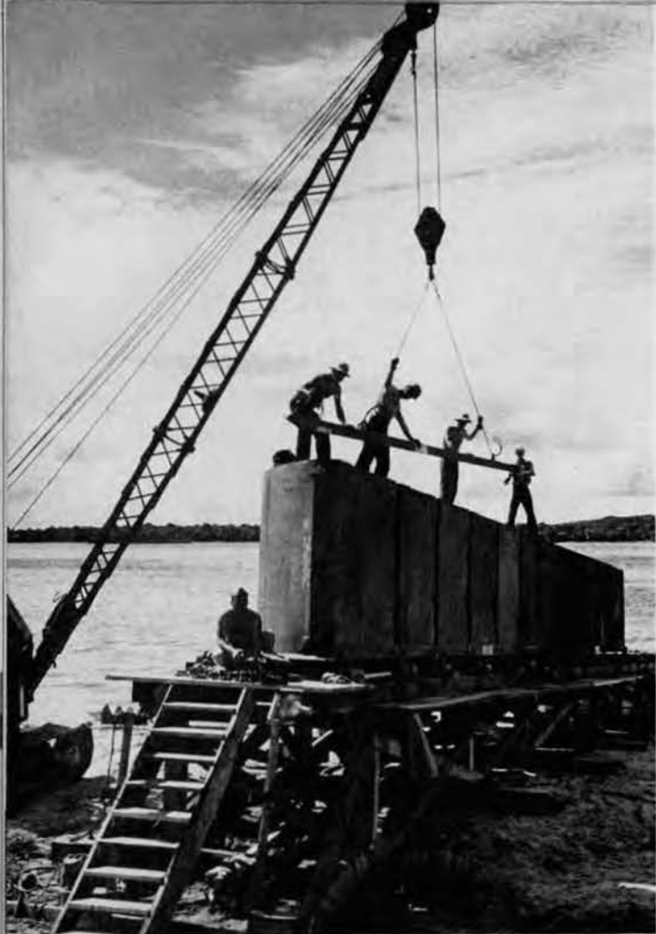
The crane makes a heavy lift that will soon be consigned to the bottom to form a foundation for permanent docks.
