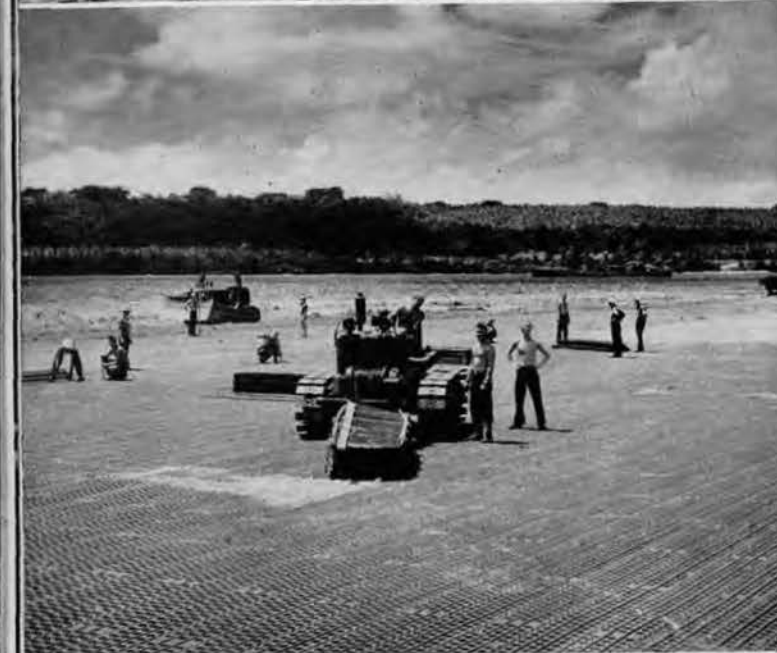
Seabees carry their roads and runways with them wherever they go. Not many days after occupying the island it was made accessible to the heaviest of land, sea and air traffic.
