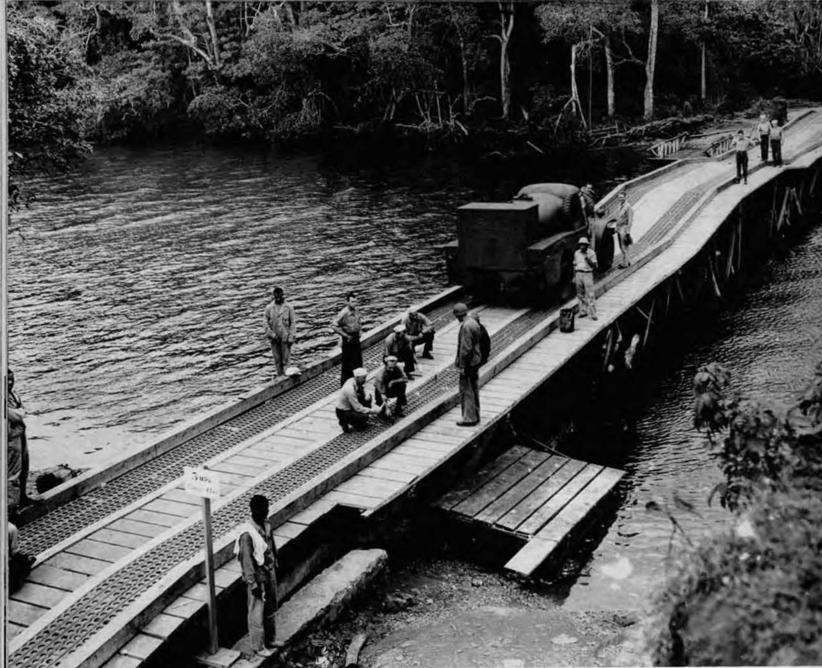
The light looking, though strong, bridge shown above is the result of expediency and ingenuity of Seabees of the 7th Battalion at war. Heavy timbers paralleling the upper surface are reinforced by steel plates forming a track which distributes the load over a larger area, over which the heaviest of equipment may cross in safety.
