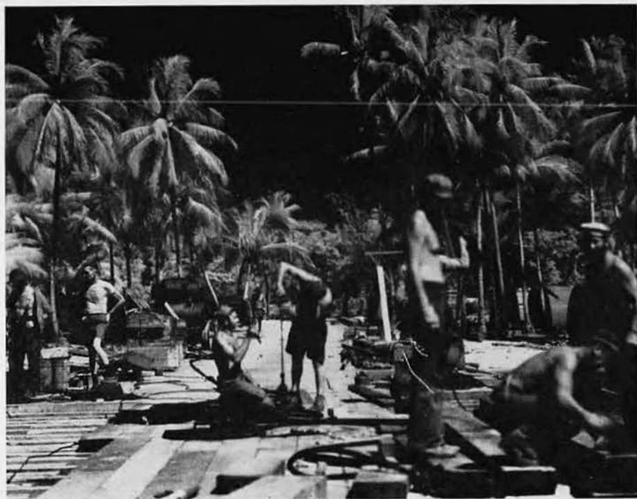
Driving piles in coral was easy, and the dock quickly began to take shape.
