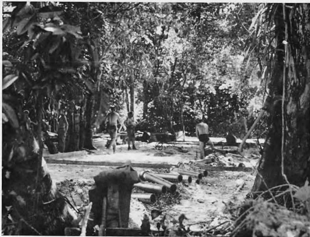
With seashells and coral sand for aggregate, tons of concrete were poured for building floors and foundations.
