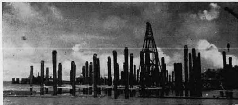
With the driving of the first pile, construction of the main dock on Mios Woendi began.
