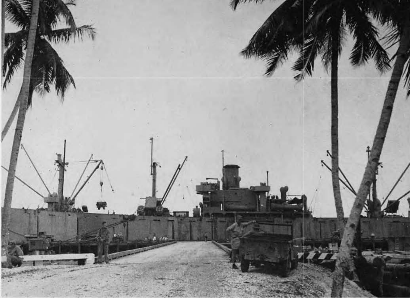
Within thirty days the dock was completed, and ships began to discharge their cargo upon it.
