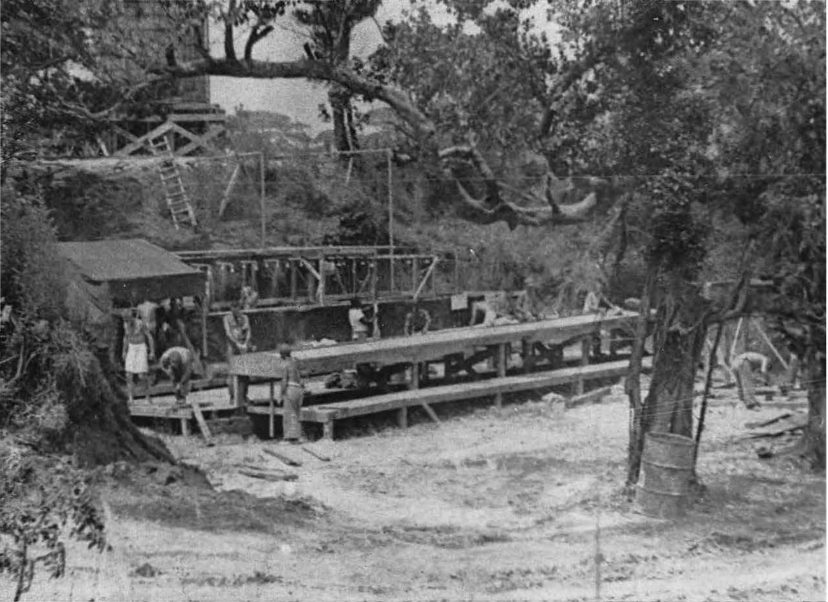
FIRST SHOWER WITH RUNNING WATER ON OKINAWA, HOT WATER, TOO; BOY, WAS IT HOT!
