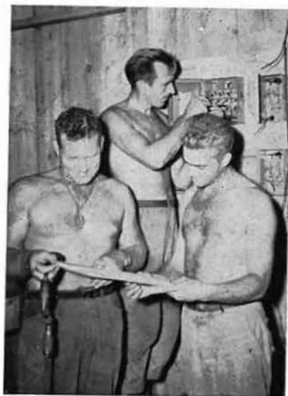
CREW WIRING CONTROL BOX
