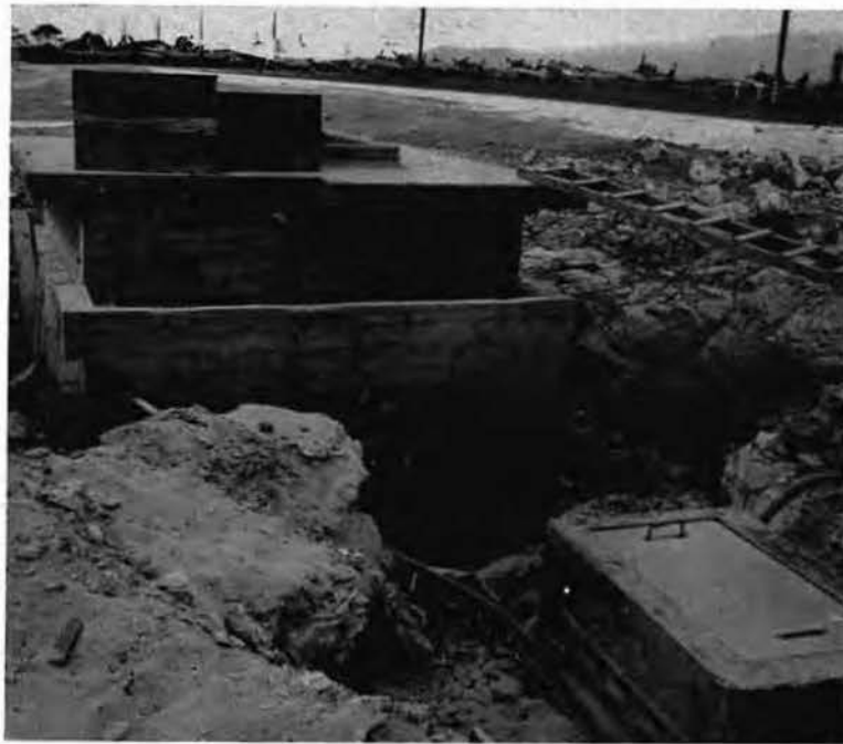
SEWAGE PUMPING STATION, EWA
