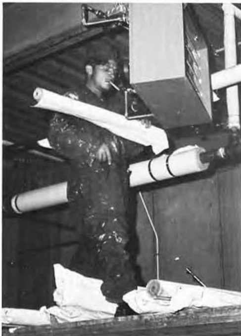
UT3 Jim Campbell works on the heating system at M-52
