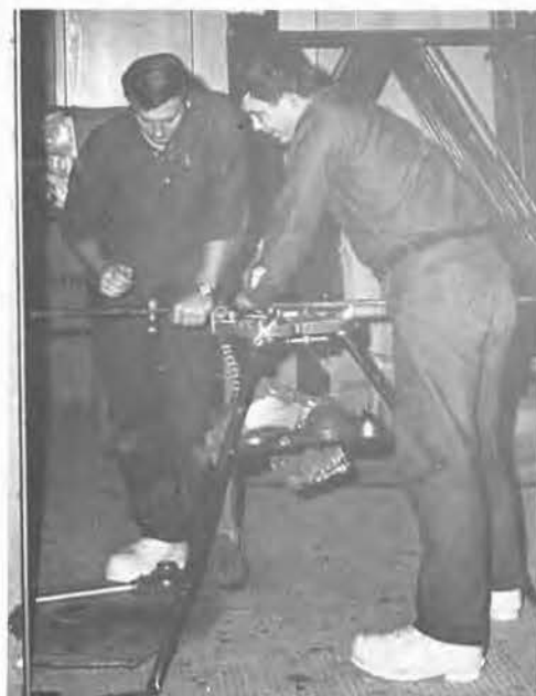
UT3 Al Templet, left, and UTCN Tuck Nipko, right, cut and thread pipe at the VXE-6 shops and offices building (M-52).
