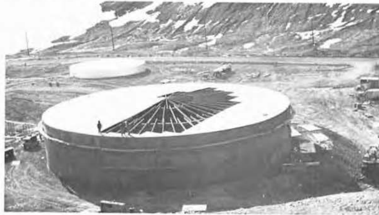
Antarctica's largest fuel tank with a two-million gallon capacity was also built this season by CBU 201.
