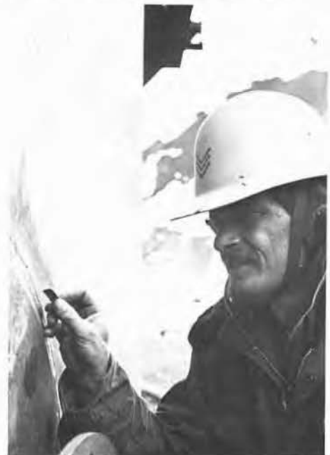
SW1 Karl Smith, Petty Officer in Charge of construction at the two-million gallon tank.
