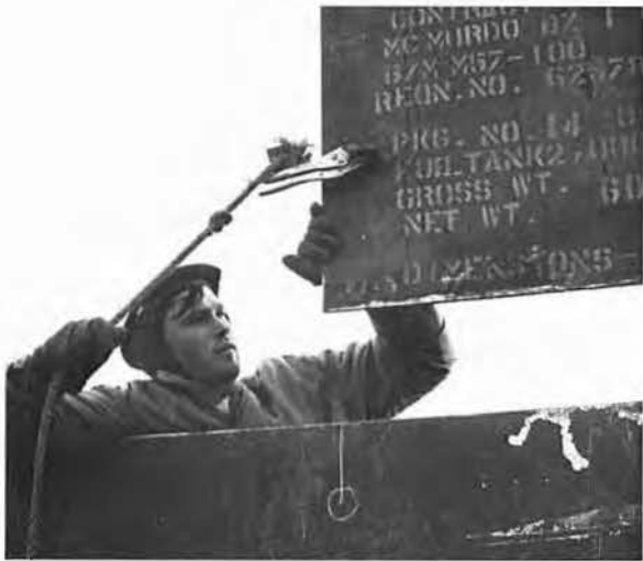
BU3 Larry Betz guides steel plate into place at the two-million gallon tank.
