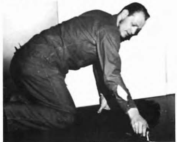
YN3 (sometimes BU) Roger Gurgul helps lay tile at personnel building (M-46).
