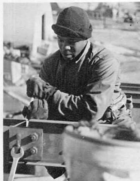
Gregory Green (top) and John Wingate (bottom) tighten Bolts on Public Works Building.
