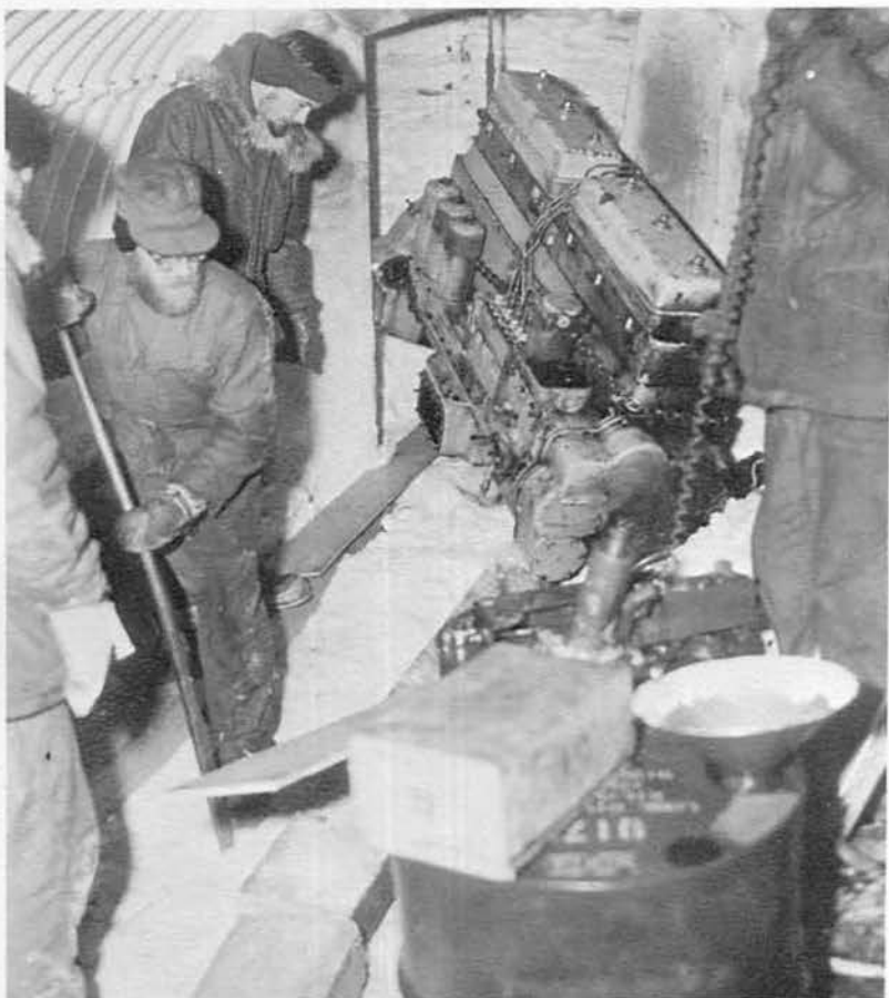
BU1 Jim Adams, CMI Paul Witte and CET3 Warren Reddick remove an old generator through the escape hatch.
