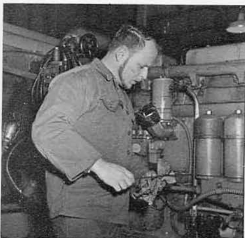
EMI Pete Rea checks the oil in a generator.
