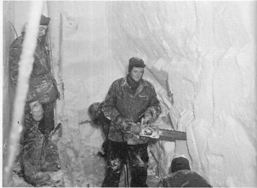
Thomas Mathers demonstrates method of shaving tunnel wall at Byrd using electric chain saw. James Cook looks on.
