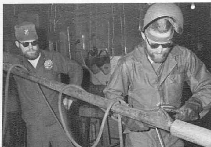
ABOVE - SF1 Robert Barker and SF1 Marion Freck weld the new flag pole.
