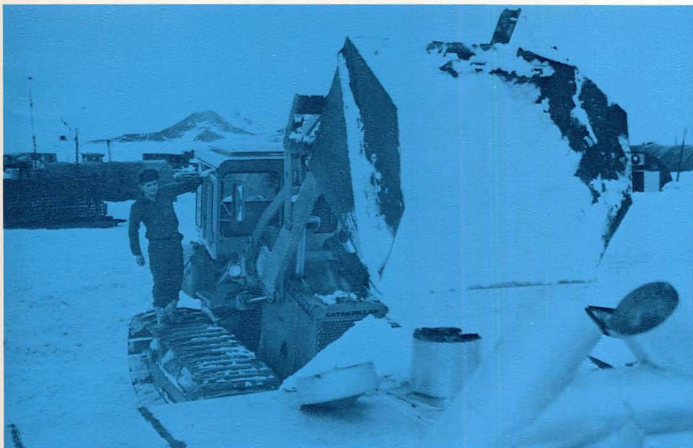
ABOVE – UTP2 Arlan W. Gooden checks the snow melter at the Strip before dumping in a load of fresh snow.
