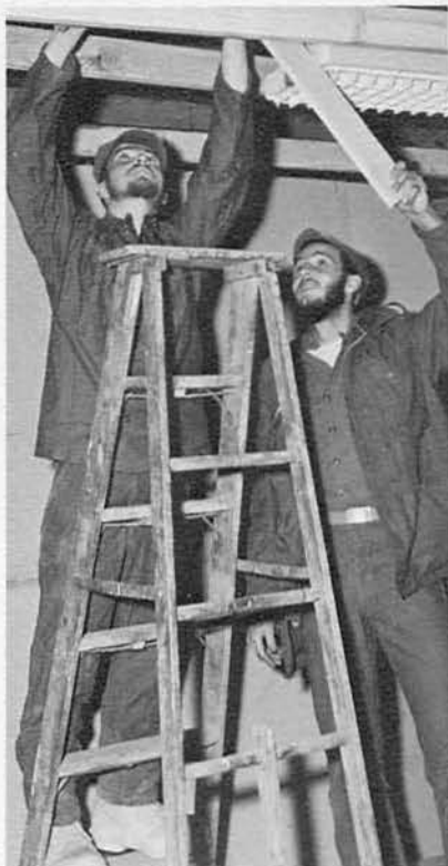
ABOVE - BULCN Richard Gendron and BUH2 David Kurre work on the new bowling alley facility.
