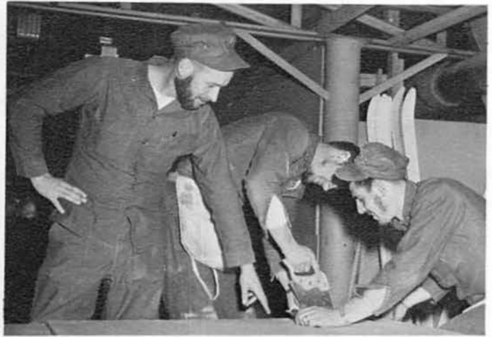
BUC Ron Cooper instructs BULCN Leslie Petrash and BULCN Stephen Zdravec in the proper method of sawing wallboard.
