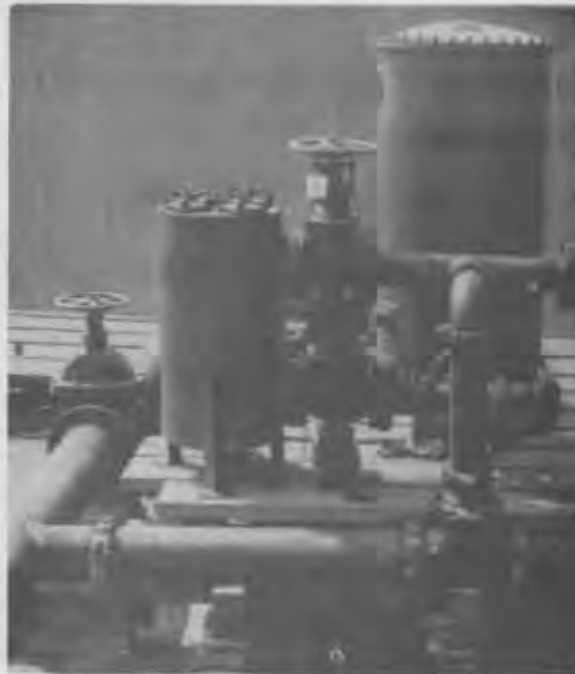
OIL CLARIFIER, FILTER UNIT (2H112)
