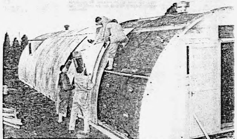
No. 1600 Seabees Erect A Quonset Hut At Camp Endicott, R. I. Official U. S. Navy Photo
