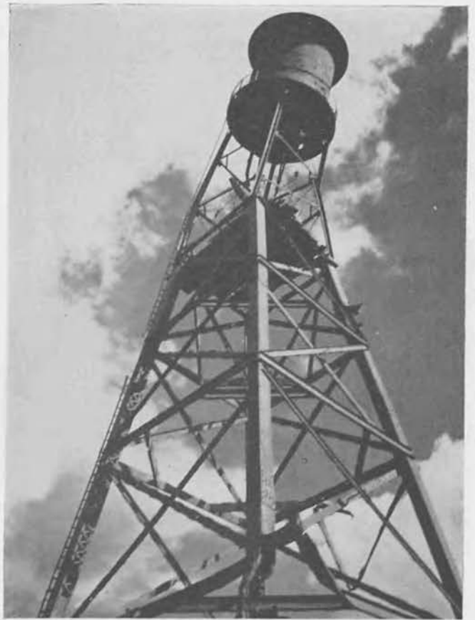
Another early project: a demolition party blasted this damaged water tower to the ground; new Island Command site.
