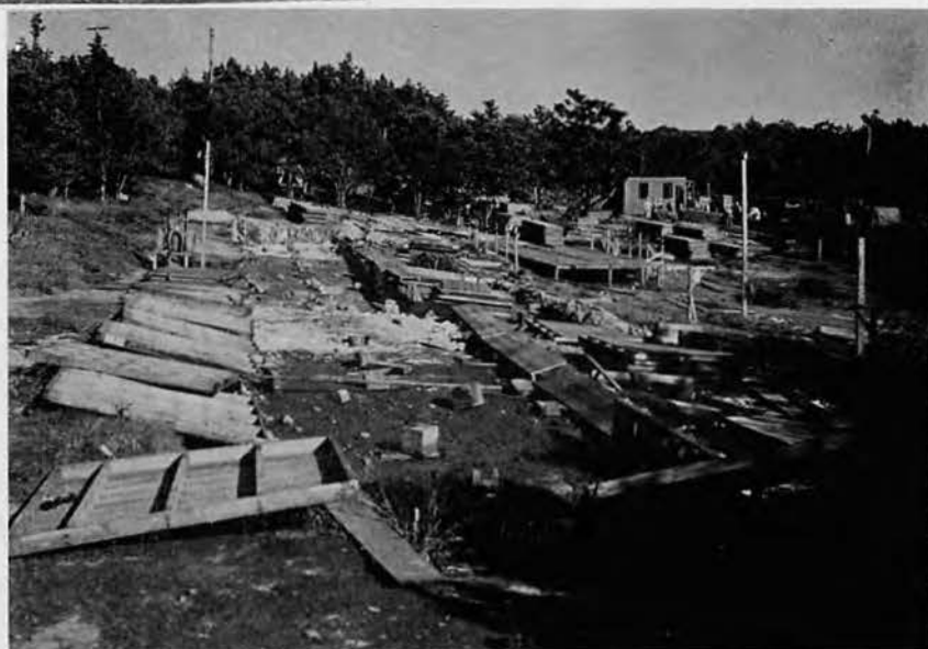
A general view of a site which only a few hours previously had been the location of several buildings. Now they have been torn down and are awaiting the loading crew.
