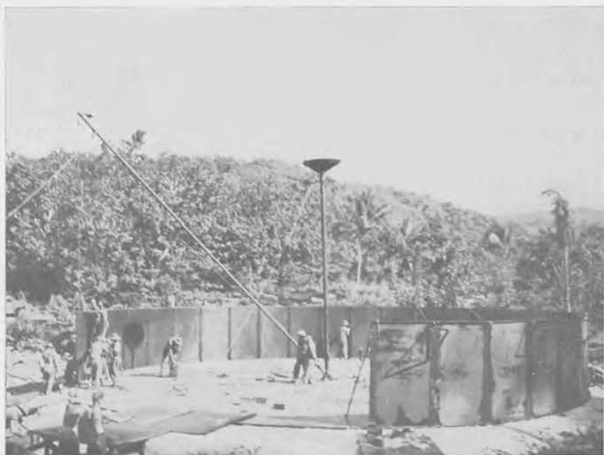
Erection of a 10,000 bbl. tank at the Assan Point tank farm. Four such tanks with connecting lines were erected at this site.
