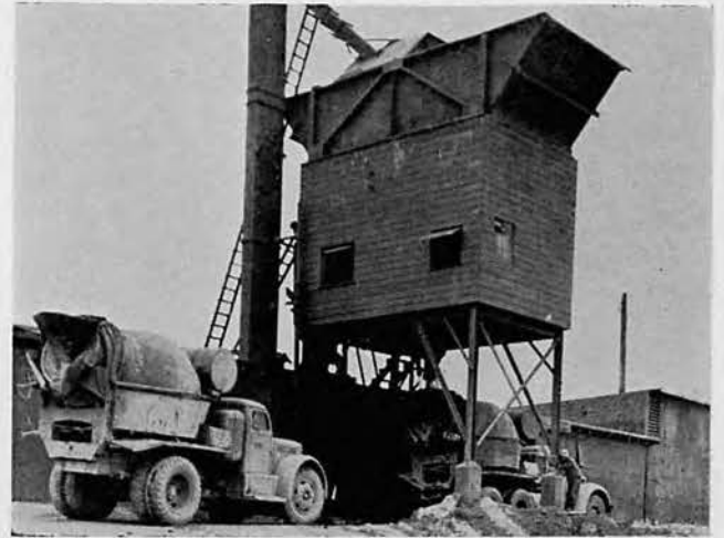
A view of the concrete plant showing one of the mixer trucks receiving its load of carefully-measured quantities of cement, rock and water.
