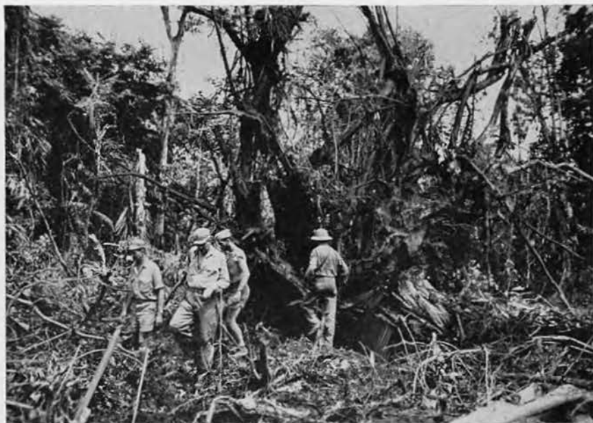
Tree roots after blasting. Comdr. Harris and Lt. Comdr. Thompson leaving site.
