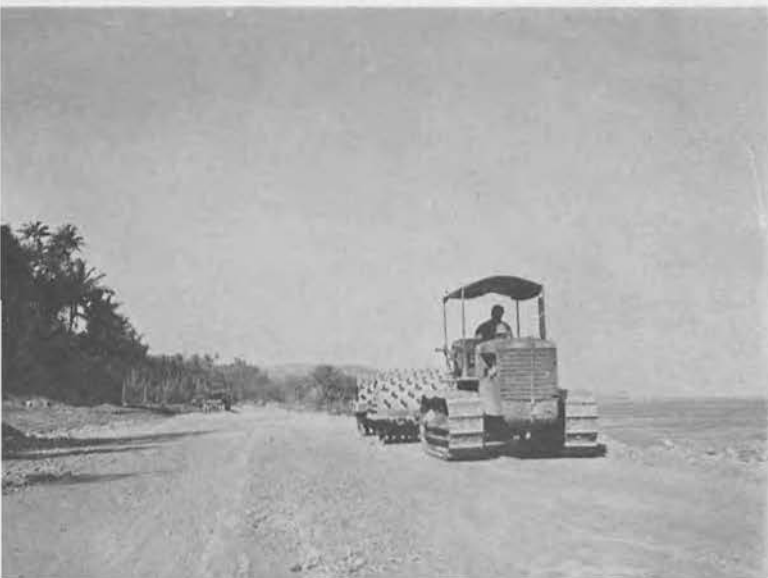
Final surfacing on the beach road between Agana and Harmon Field. Site of the Fifth Naval Construction Brigade Headquarters shows on the horizon to the right of the tractor.
