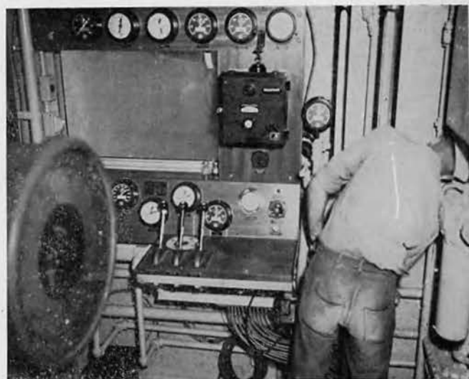
This complicated installation was put in by the 49th in the engine test cell and was used in the control and testing of engines.
