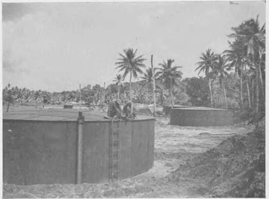
Tumon Bay tank farm. Two 10,000 bbl. and twenty 1,000 bbl. tanks with connecting lines were erected by the 53rd NCB. This was a part of the storage for AvGas for B-29's.
