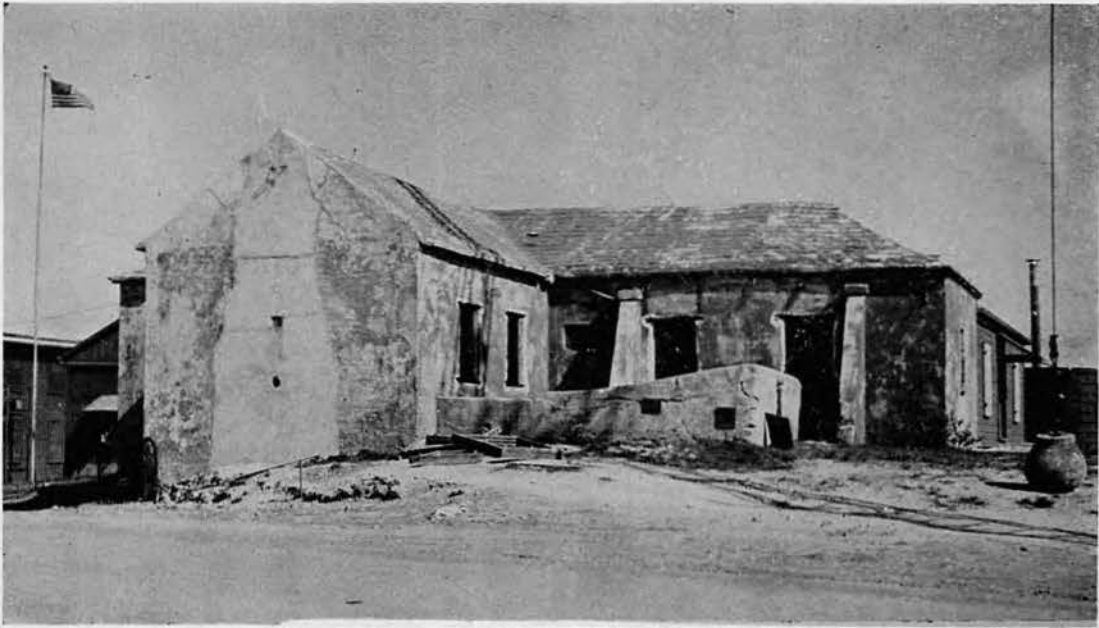
This old Bermuda residence which was in the Marine barracks area was used for a long time as the Marines' Post Exchange. It was decided, however, that a newer and more modern building was needed so the old place was torn down.
