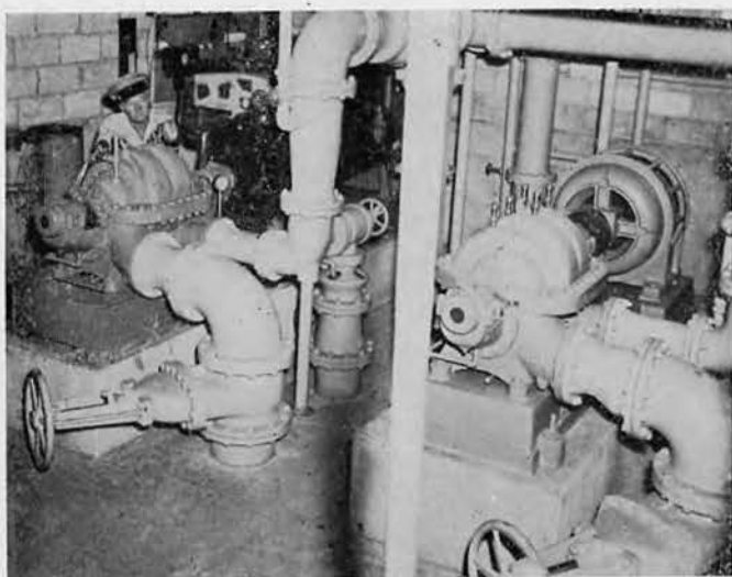
Chief Schaeffer checks a pump in the evaporator plant. The base depended a great deal upon this plant to supply fresh drinking water manufactured from sea water.
