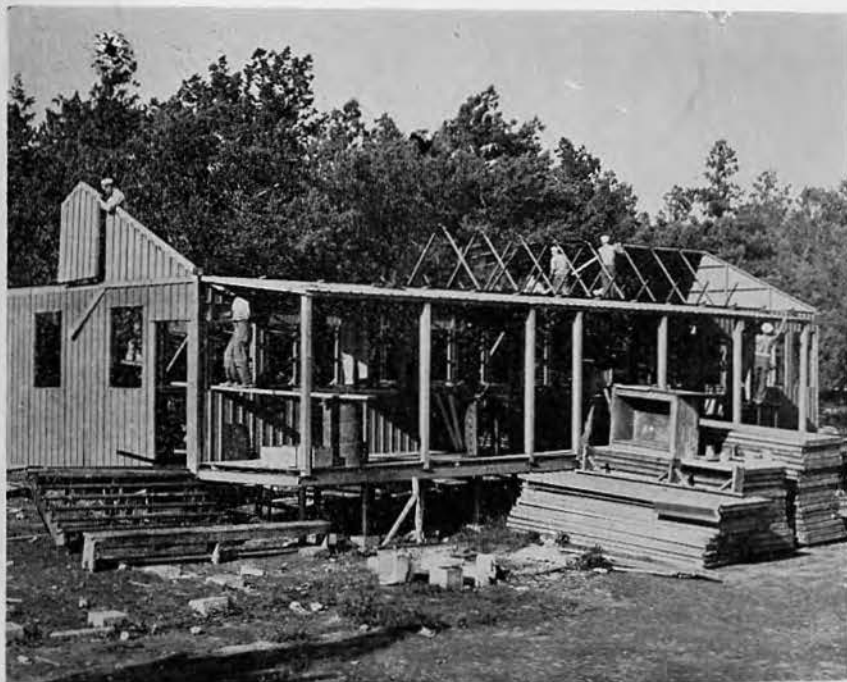
Battalion workers made quick work of these buildings, dismantling them and re-erecting them in short order. Virtually a small city had to be torn down and put up again in a new location.
