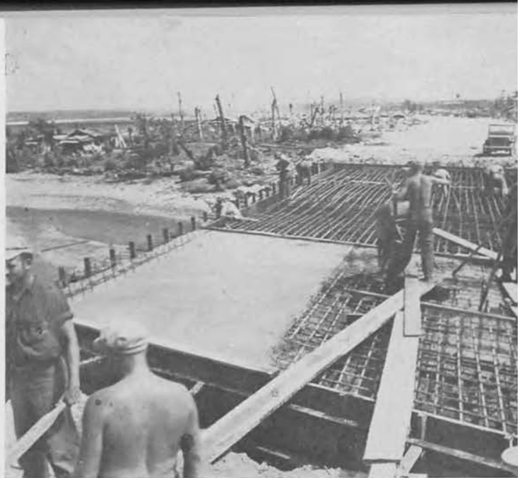
This structure over Anigua River near the Agana Cemetery is a reinforced concrete deck supported on wood piling. Note shattered palm trees in background.
