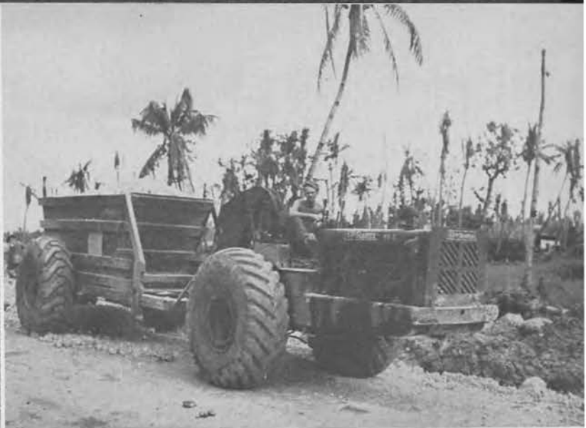
Spreading the coral base course on the Sumay-Piti Road Crocher at the controls of the tourne-trailer.
