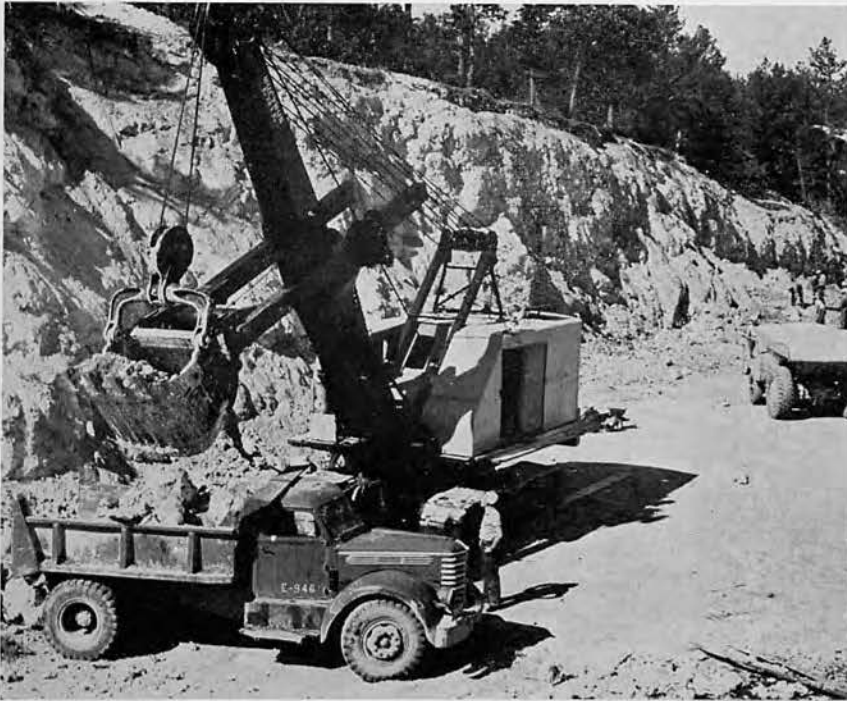
Great quantities of solid limestone rock had to be moved to make way for roads and buildings. The rock was crushed and processed and then used for making concrete and building roads.
