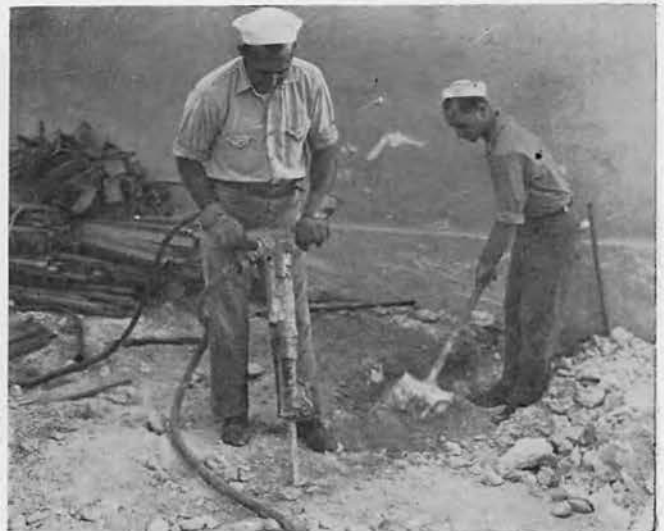
Even with all the earth-moving equipment at hand there was still a lot of hand work to be done. Some day an ingenious Seabee will probably invent a machine which will forever do away with jackhammers and shovels. (He'll probably get a medal for it, too!).
