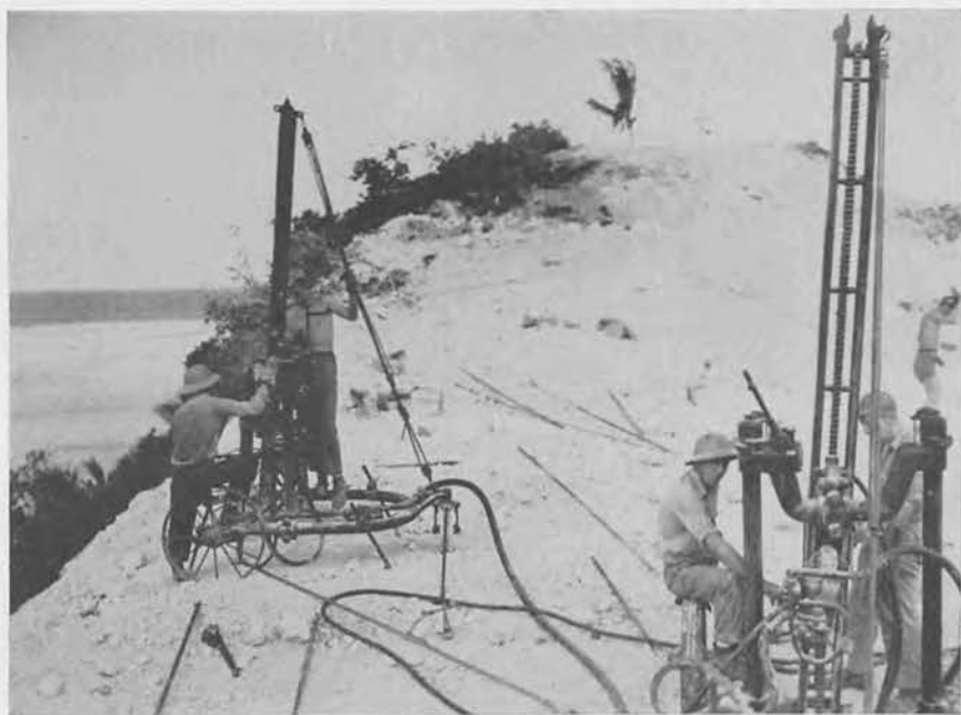
Wagon Drills in initial operations on the 115' Assan Point cut. Approximately 200,000 cu. yds. of excavation came from this site.
