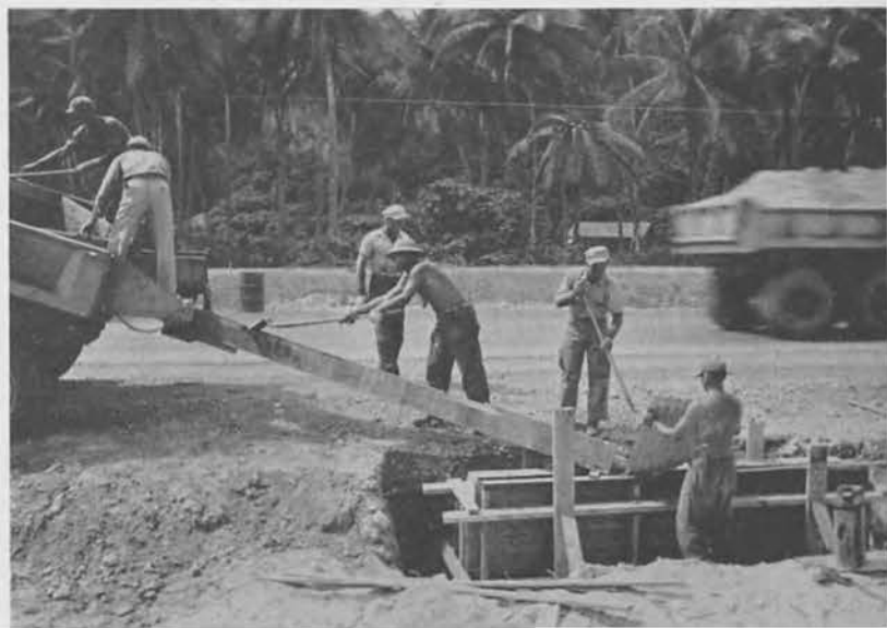
Pouring culvert headwalls on the beach road between Agana and Harmon Field.
