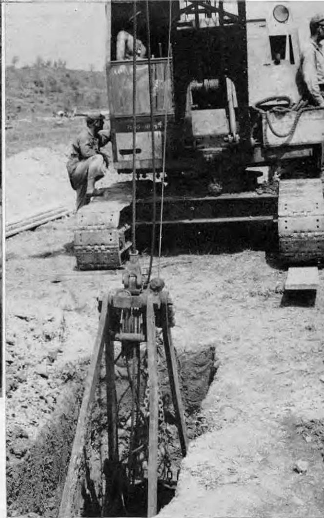
Top: Further improvisation of the oil drum. At Right: Digging latrine pits by "Clamshell." Below: Showing the use of oil drums and coconut logs in the construction of a large capacity culvert.
