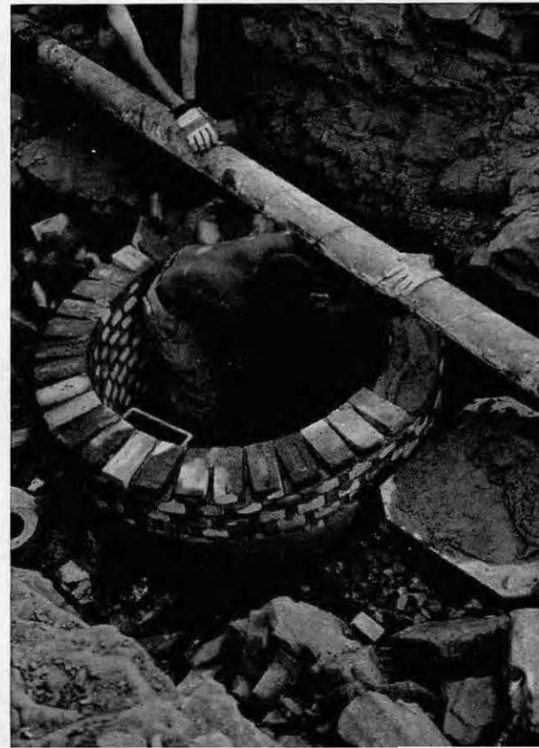
And how about those back-breaking man holes. The hot sun bearing down made that work a torture, but it had to be done.
