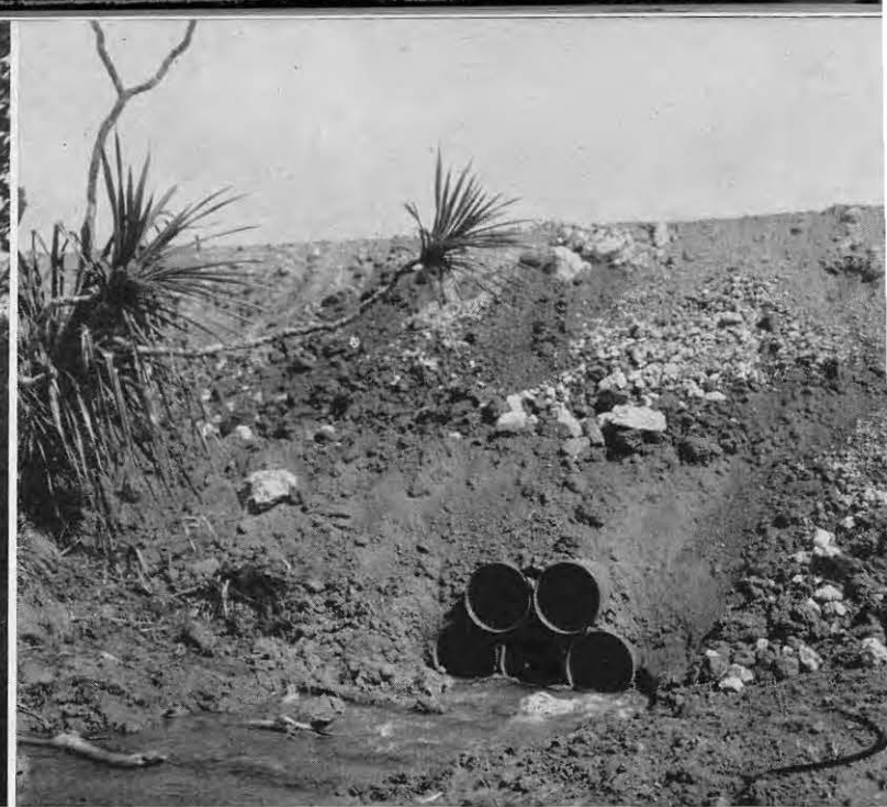
Oil drum culvert under a fourteen-foot fill on one of the N. A. D. roads.
