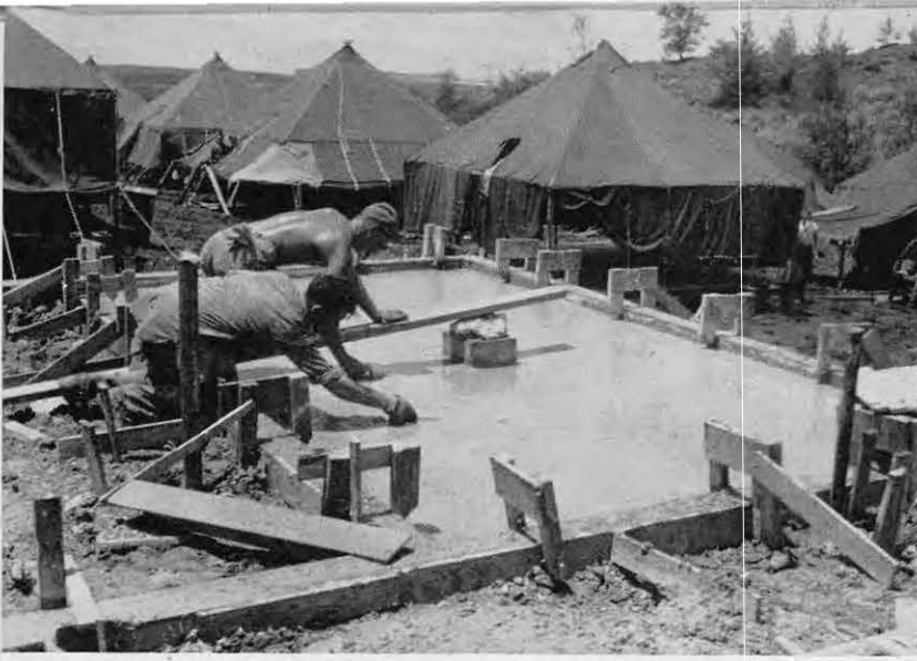
Peterson and Barney Convey putting the finishing touches on one of the shower floors. Barney was one of those rare persons that never needed to be reminded about there being a war on, and was one of the battalion's hardest and most conscientious workers.
