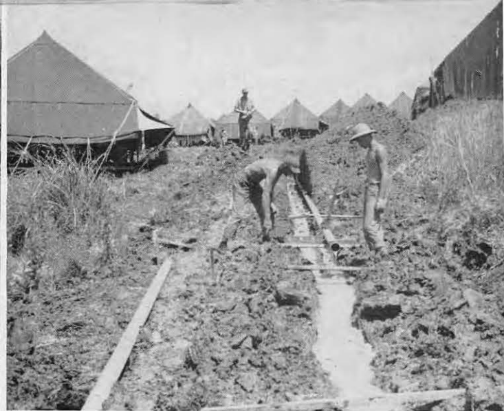
The rainy season made laying pipe lines anything but a pleasant. Almost as soon as the ditches were dug, the skys would let down deluge, caving in the sides and filling the ditches with that wet s
