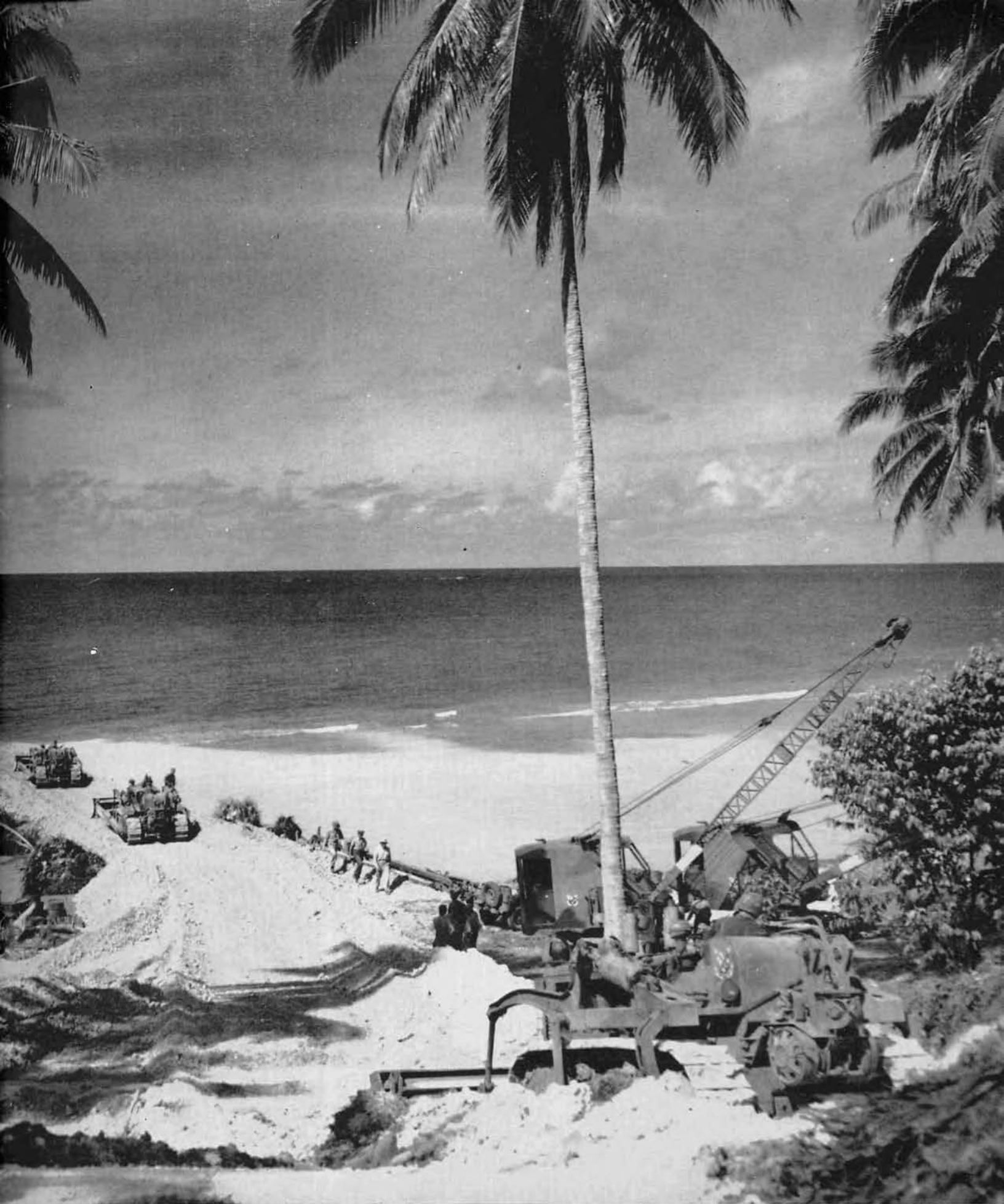
Bulldozers clear a road to the site where a dock will be built on Emirau Island, to facilitate unloading of LSTs (Landing Ship, Tank).
