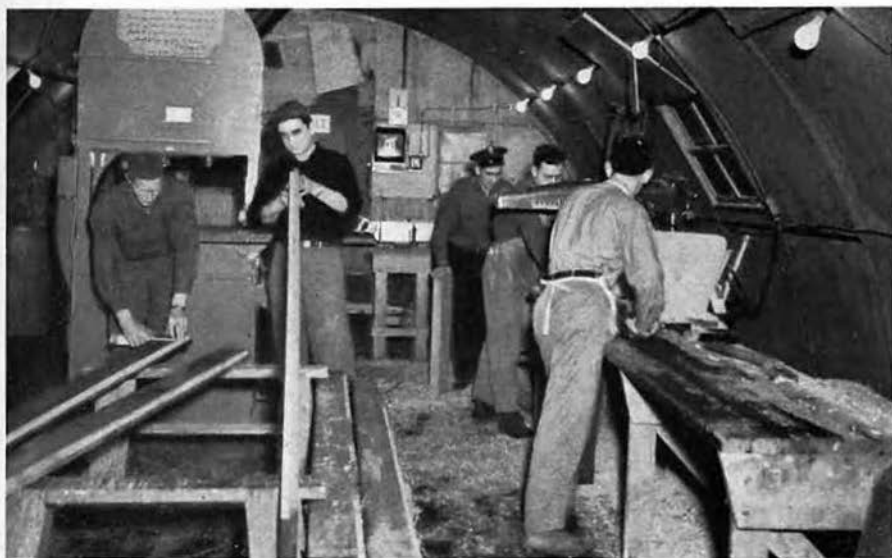
SHOP MEN or outside crews, the carpenters were always busy . . . furniture or warehouses . . . Quonsets or bowling alleys . . . storm shelters or jeep bodies . . . these craftsmen turned them out.
